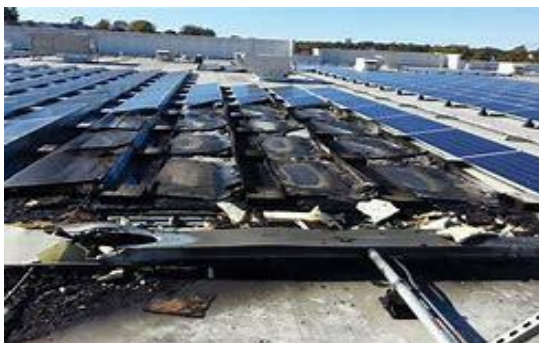
Remains of a solar panels fire
