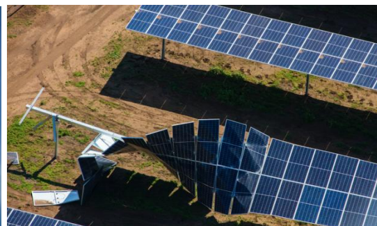
Oakey 2 wind damage
