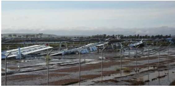
Storm damage to a PV solar IEGP
