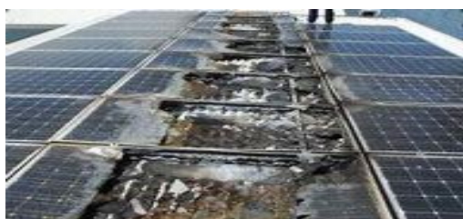
Fire shuts down whole solar array
