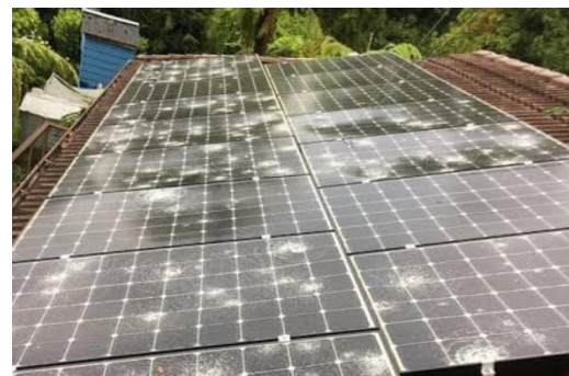
Solar panels damaged by hail
