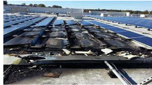
Fire damage to a PV solar IEGP
