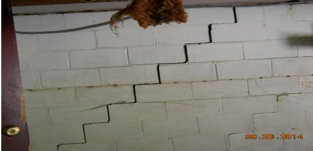
Home subsidence due to mining:
