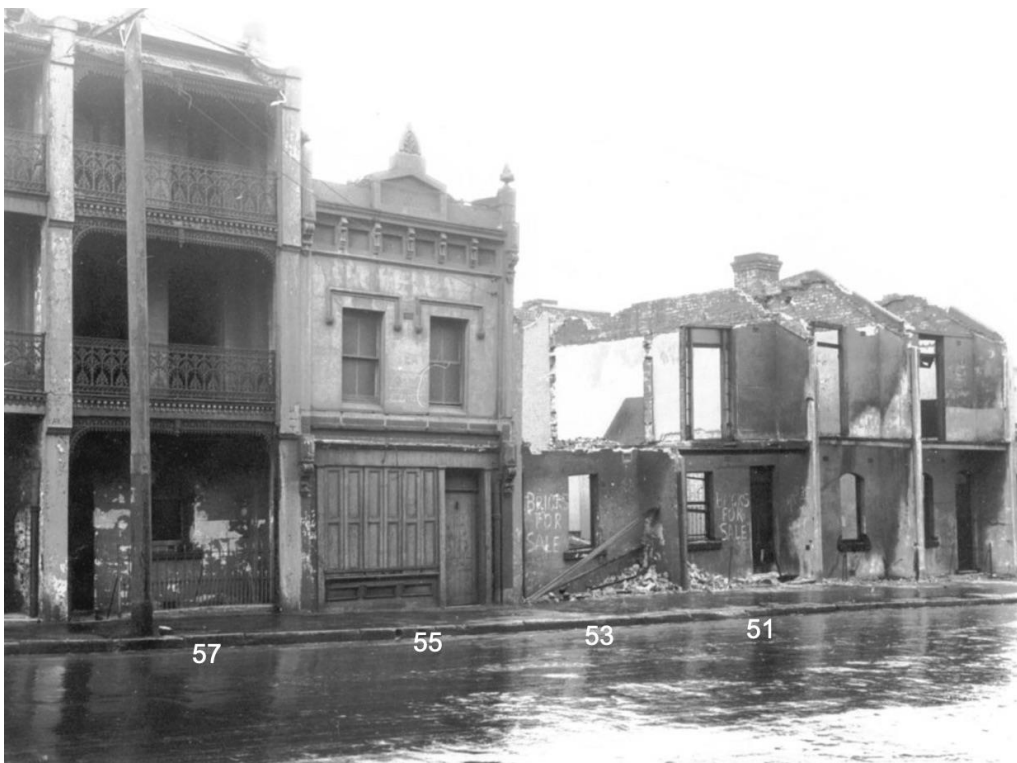
Figure 84: 20 October 1930 – Shops and houses being demolished at Union Street, near corner of Edward Street. Shop at 55 Union Street bearing date 1881 (Source: City of Sydney Archives, Shop and houses being demolished (20/10/1930), [A-00037643]. https://archives.cityofsydney.nsw.gov.au/nodes/view/664010 )
