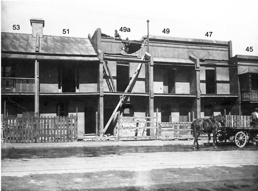
Figure 75: 8 September 1916 – Photograph of dwellings at 47-59 Union Street, Pyrmont, with workers working on the parapet. From Demolition Books. In c1905, these terraces replaced the former hall which was once located at 49/49a Union Street, before being gutted by fire in 1903. It is unclear what works were carried out to the terraces at that time, as double storey houses continued to be located at the site until the early 1930s (Source: City of Sydney Archives, Dwellings, Union St (47-59), Pyrmont, 8 September 1916 (08/09/1916), [A-00036813]. https://archives.cityofsydney.nsw.gov.au/nodes/view/663180 )
