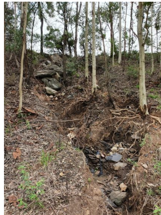
Photograph 47– Area 5/6: Speedway western boundary embankment (gully erosion exposing subsurface materials)
