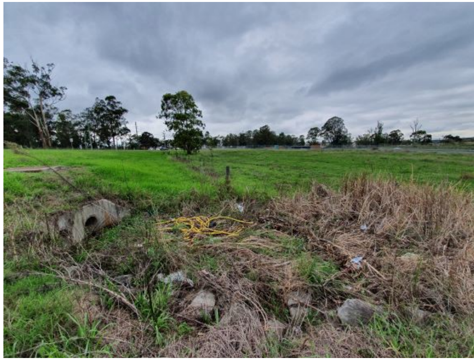
Photograph 49 – Area 7: Worksite facilities and amenities – Culvert crossing Ferrers Road from Area 6 discharging to Area 7 (facing south)
