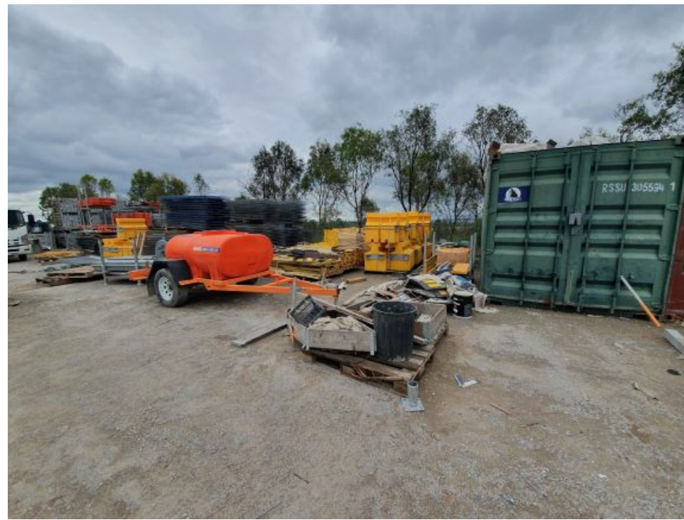
Photograph 26 – Area 4: Carpark D – Coates Hire storage area containers and trailers (facing west)
