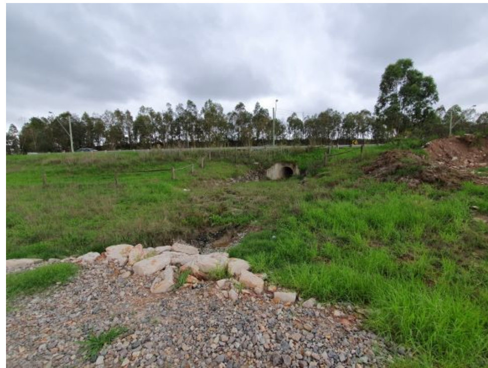
Photograph 53 – Area 7: Worksite facilities and amenities – Culvert crossing Ferrers Road from Area 6 discharging to Area 7 and Eastern Creek (facing north-east)
