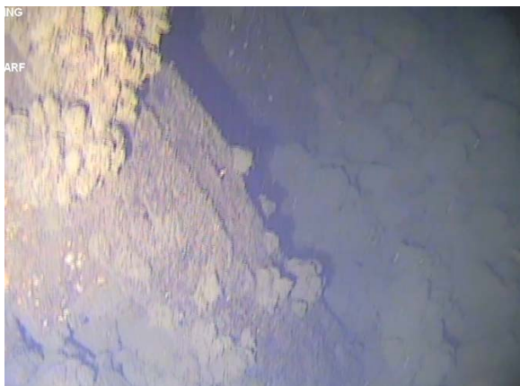
Figure 100: Two of the cut off timber piles near the southern 'E' steel pile. (Image from T10 (a) Cockle Bay 210705; 07:39).
