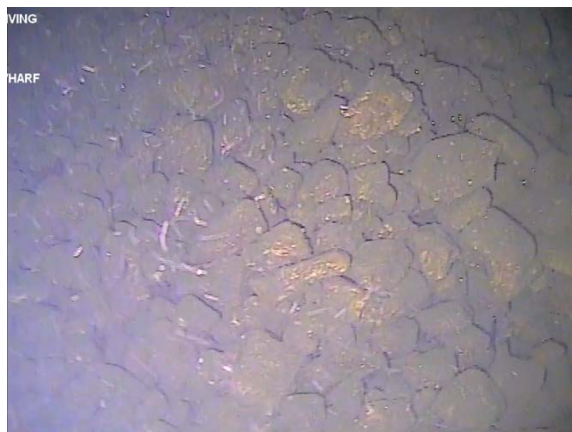
Figure 61: Rock embankment at eastern end of T2. (Image from T2 (a) Cockle Bay 210705, 06:39).
