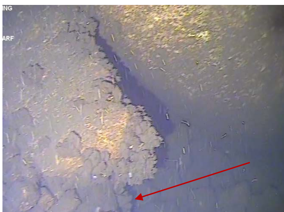
Figure 102: Rectangular piece of concrete leaning against southern 'E' pile. Timber pile underneath indicated by red arrow. (Image from T10 (a) Cockle Bay 210705; 09:01).
