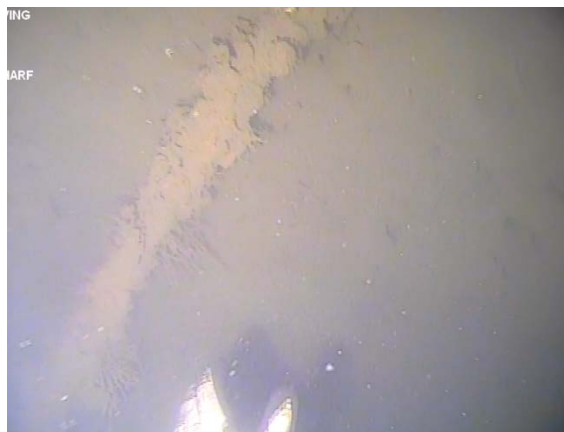
Figure 65: Ferrous pipe running northwest to southeast across the centre of the bent. (Image from T3 (a) 210705, 03:05).
