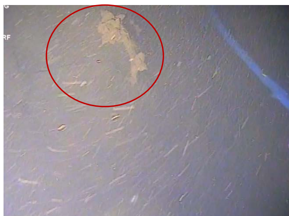
Figure 103: Top of the northern cut off timber pile closest to the northern 'E' steel pile. Note heavy deterioration. (Image from T10 (b) Cockle Bay 210705; 02:52).
