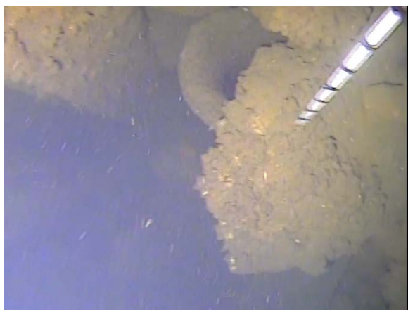
Figure 90: Degraded and hollowed out timber pile northeast end of transect 7. (Image from T7 (b) Cockle Bay 210705; 03:56).
