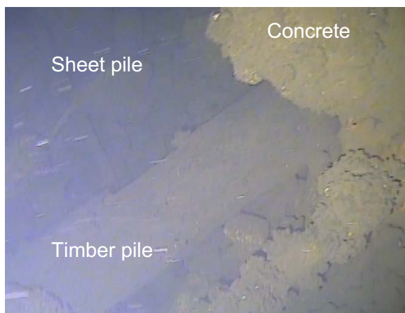
Figure 89: Horizontal timber pile on the northeast end of T7. (Image from T7 (b) Cockle Bay 210705; 03:38).
