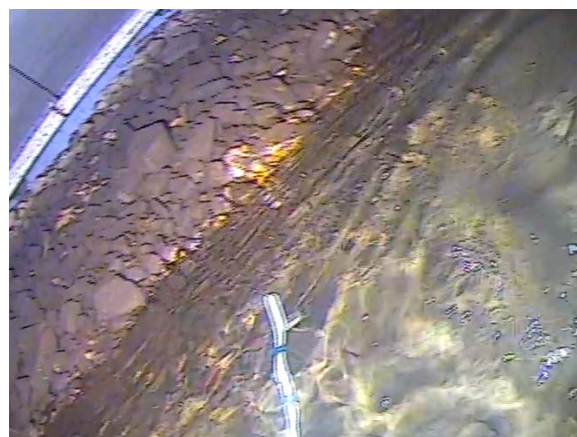
Figure 106: Rock embankment at eastern end of T11. (Image from T11 (a) Cockle Bay 210705; 03:11).
