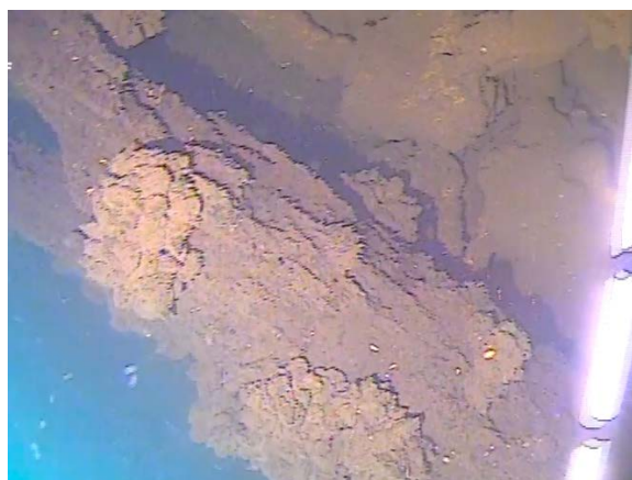
Figure 98: Loose fallen pile next to northern 'B' pile. (Image from T9 (a) Cockle Bay 210705; 05:22).
