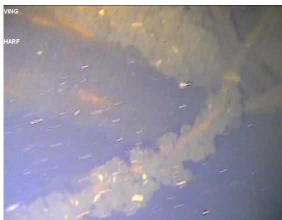
Figure 69: Sheet piling in background with loose ferrous piping in the foreground. (Image from T3 (a) Cockle Bay 210705, 07:38).
