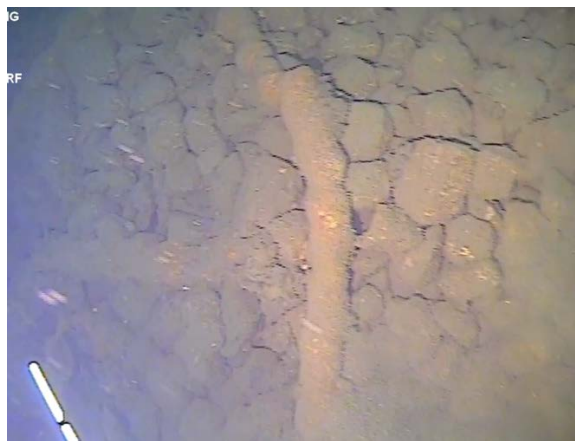
Figure 96: Scattered ferrous piping lying on top of the rock batter. Rocks measuring 100 - 300 mm in size. (Image from T9 (a) Cockle Bay 210705; 01:45).
