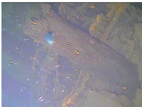
Figure 97: Timber pile adjacent to 'B' pile in centre of bent and surrounded by construction debris. (Image from T9 (a) Cockle Bay 210705; 03:06).
