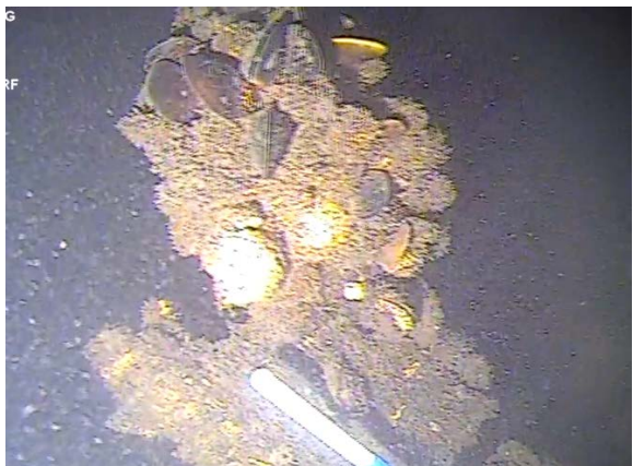
Figure 104: Heavily deteriorated cut off timber pile 1500 mm to the south of the northern 'E' pile. (Image from T10 (b) Cockle Bay 210705; 05:00).
