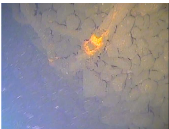
Figure 88: Construction debris resting on top of the rock batter at the eastern end of the transect. (Image from T7 (b) Cockle Bay 210705; 02:45).
