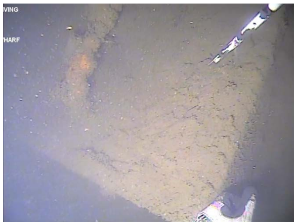
Figure 62: Mooring block northern side T2. (Image from T2 (a) Cockle Bay 210705, 08:29).
