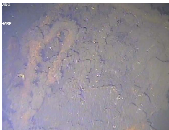
Figure 73: At the eastern end of the bent, on the rock batter, there is construction debris, consisting of ferrous pipes, possible service pipes and/or scaffolding. (Image from T4 (a) Cockle Bay 210705, 05:46).
