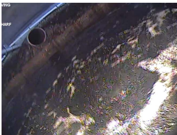
Figure 72: Stormwater at eastern end of bent. (Image from T4 (a) Cockle Bay 210705, 05:13).
