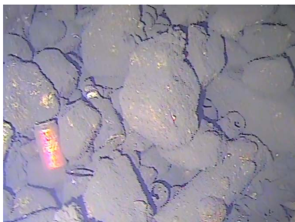
Figure 105: Example of rock batter at ‘C’ pile. (Image from T11 (a) Cockle Bay 210705; 02:42).
