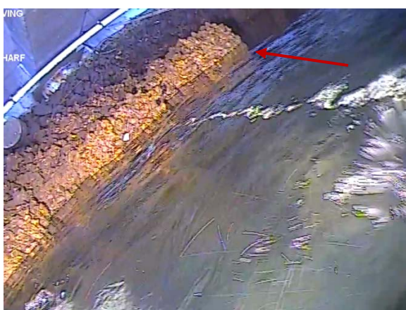
Figure 74: Sheet pile wall 1.5 m behind 'D' pile. The sheet pile returns to the east to run into the sea wall at the red arrow. (Image from T4 (a) Cockle Bay 210705, 07:06).
