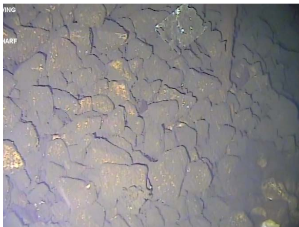
Figure 55: Example of rock embankment at western end of T1, slope of 45°. (Image from T1 (a) Cockle Bay 210705; 07:10).
