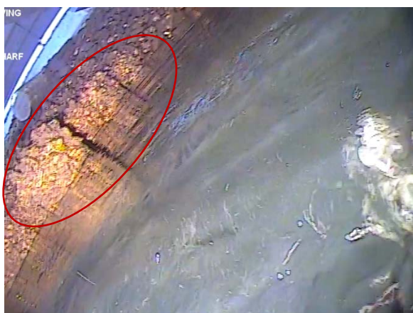
Figure 68: Sheet piling appears to start in this bent. (Image from T3 (a) Cockle Bay 210705, 07:49).
