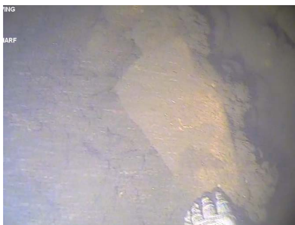
Figure 66: Large piece of concrete resting on the rock batter. (Image from T3 (a) Cockle Bay 210705, 06:14).
