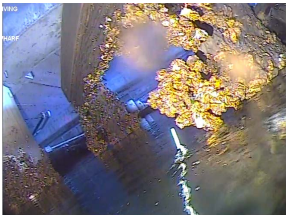
Figure 58: Timber stormwater baffle; 'D' pile to the left of image. Note large hole in net and missing timbers from baffle. (Image from T2 (a) Cockle Bay 210705, 03:57).
