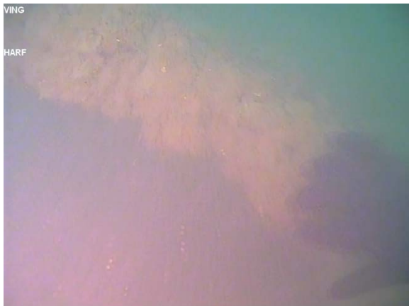
Figure 94: Rectangular pile on a 45° angle to the south in the centre of the bent adjacent to 'A' pile at the western end of T8. (Image from T8 (d) Cockle Bay 210705; 08:07).
