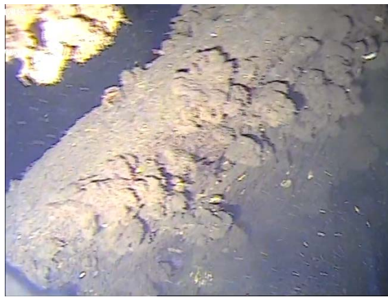
Figure 59: Example of timber planking for stormwater baffle. (Image from T2 (a) Cockle Bay 210705), 04:37).
