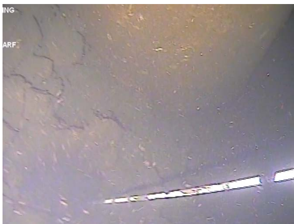
Figure 82: The rock batter is exposed at the 'C' pile. (Image from T6 (a) Cockle Bay 210705; 04:10).
