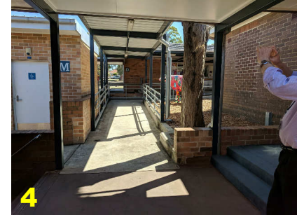
COVERED WALKWAYS & PATHS LINKING BUILDINGS BUT INSTANCES OF DISABILITY ACCESS NON COMPLIANCE.
