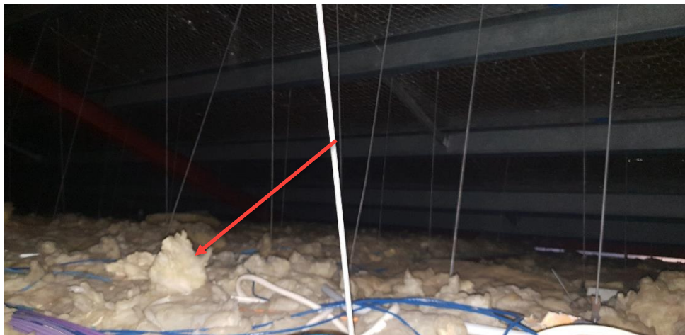
Photograph 1: B00A - Ceiling space – SMF ceiling batts
