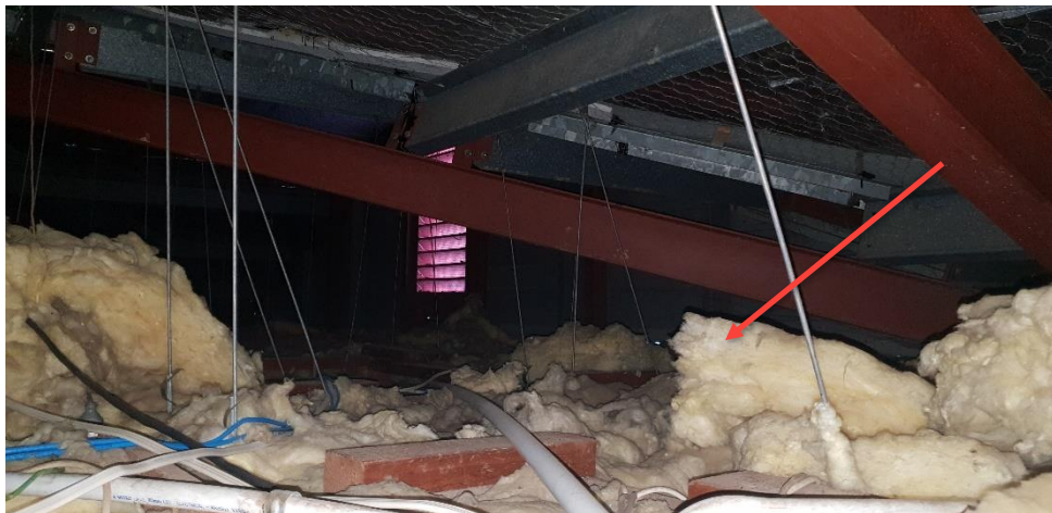
Photograph 3: B00A - Ceiling space – SMF ceiling batts
