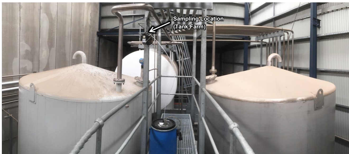
Photo 2 Tank Farm (Storage) Sampling Location
