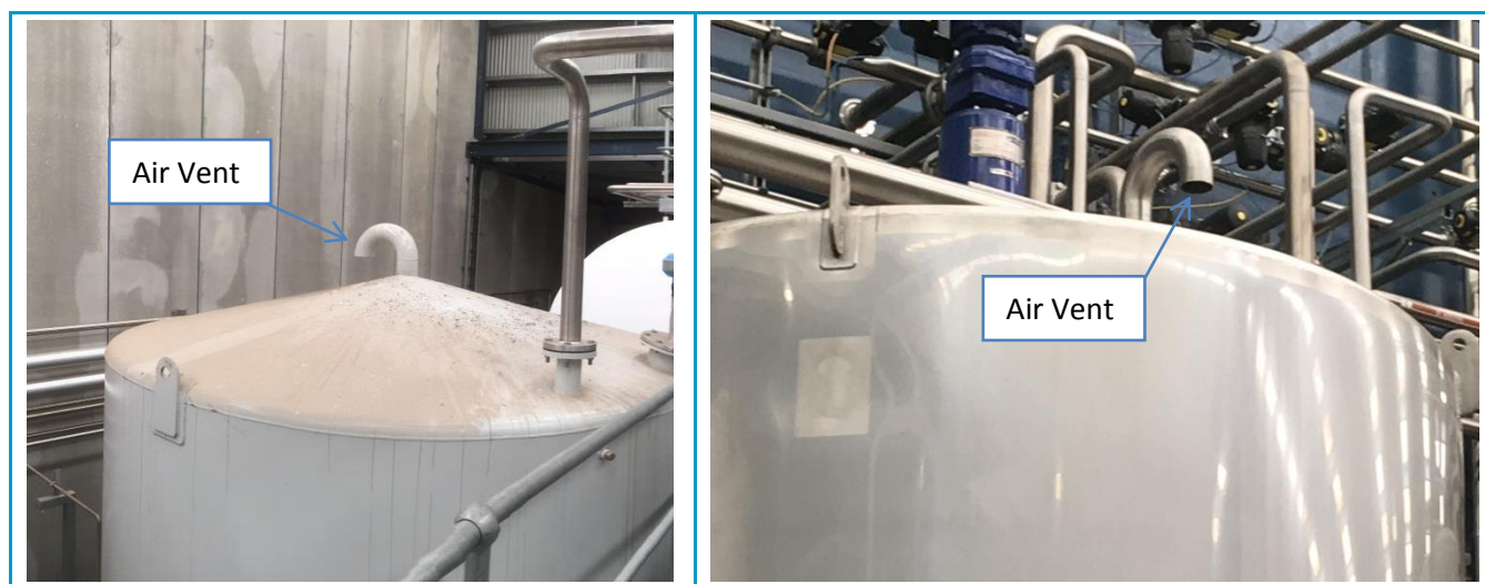
Photo 1 Vent Type for Storage and Blending Tanks
