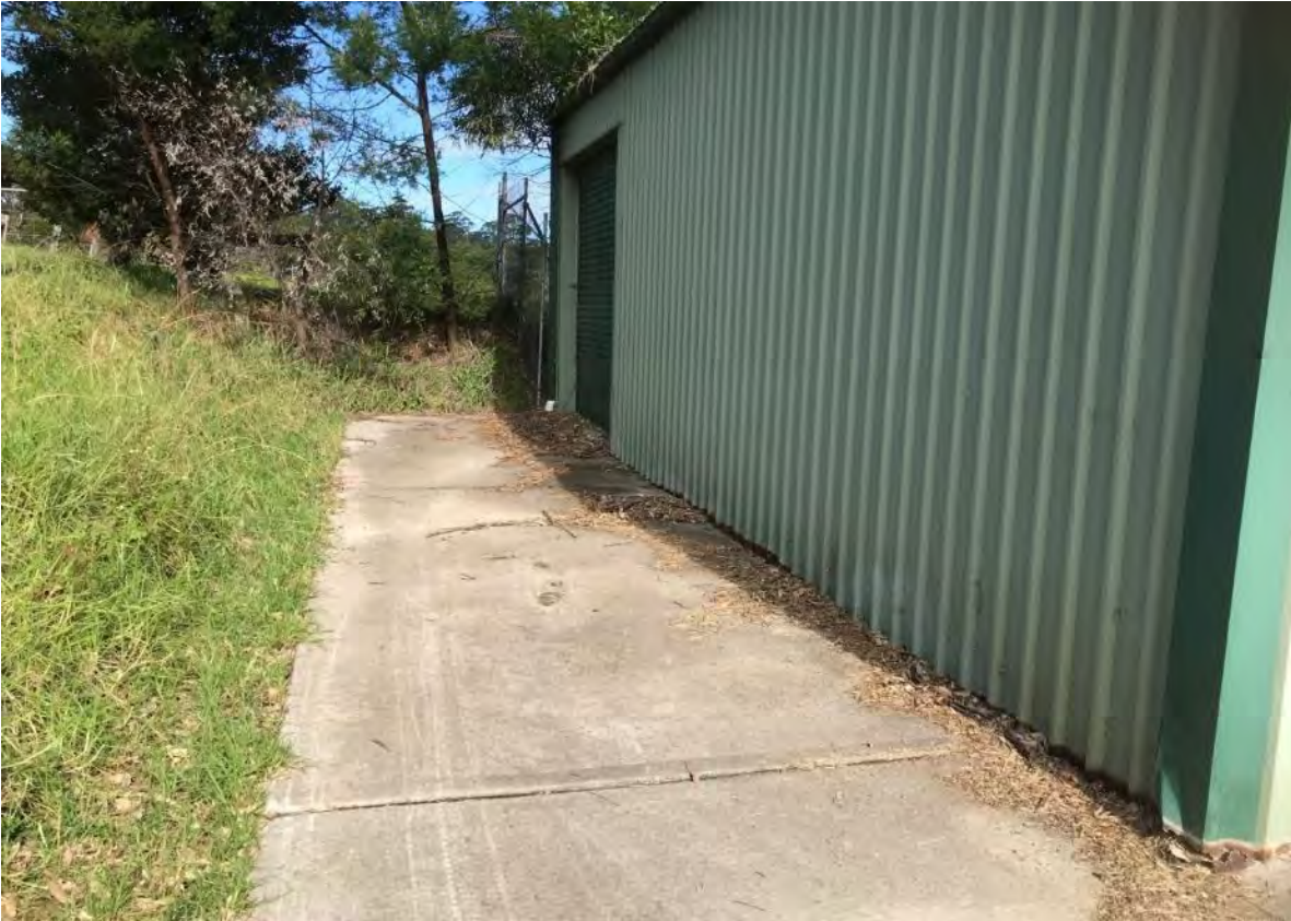
Photograph 11: the condition of a concrete slab surrounding the shed located in the south eastern portion of the site
