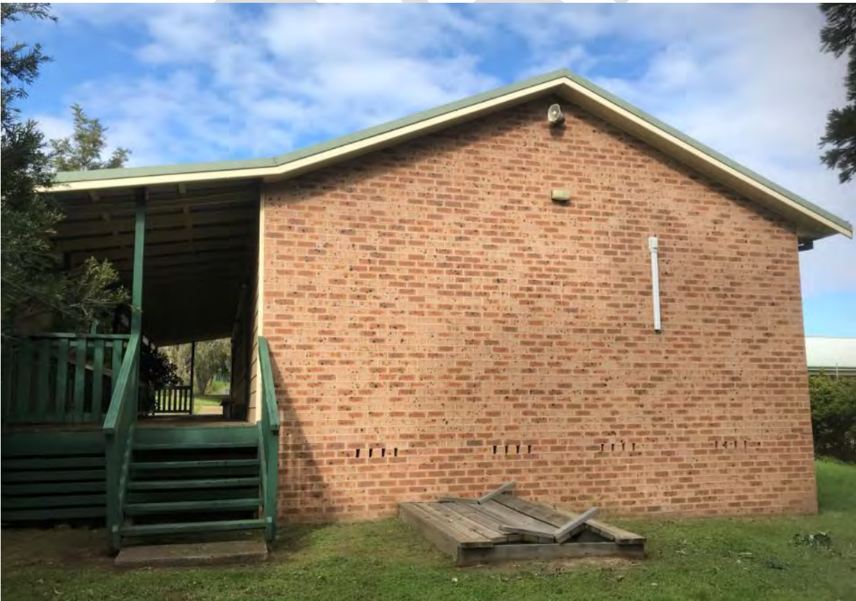
Photograph 24: a building within the proposed SSP redevelopment footprint that is proposed for demolition
