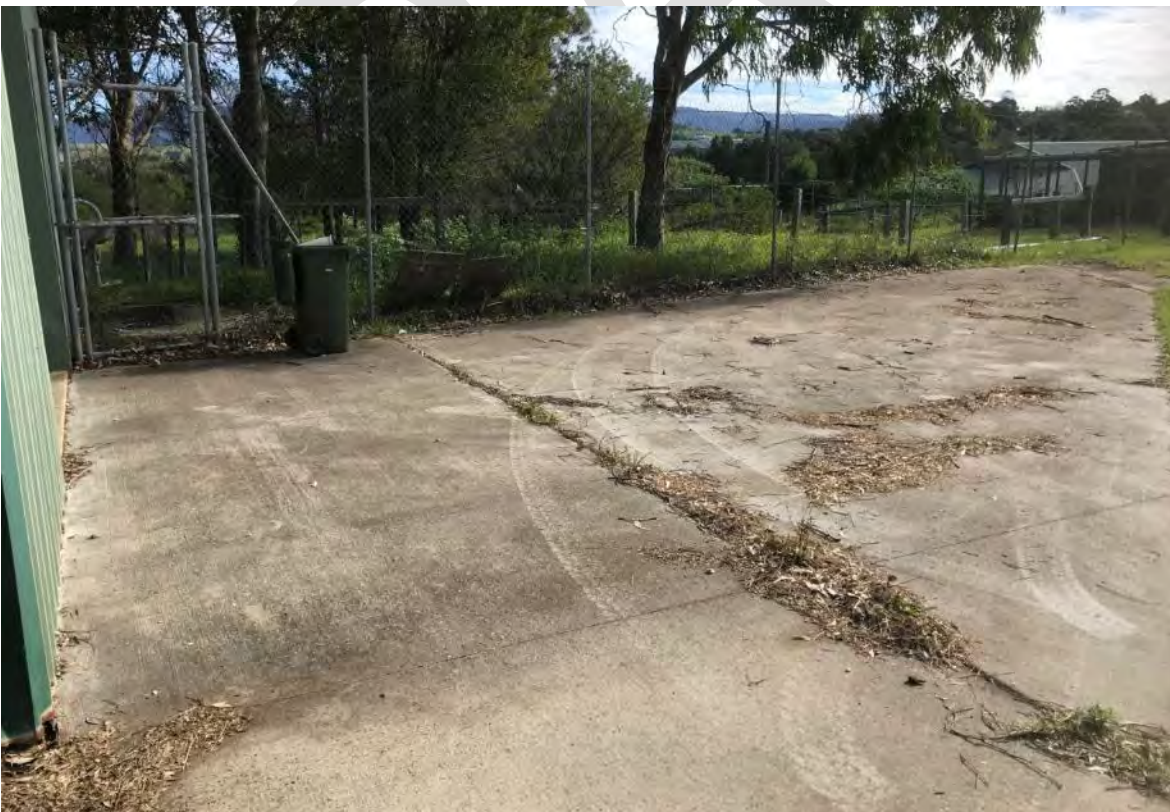
Photograph 12: the condition of a concrete slab surrounding the shed located in the south eastern portion of the site
