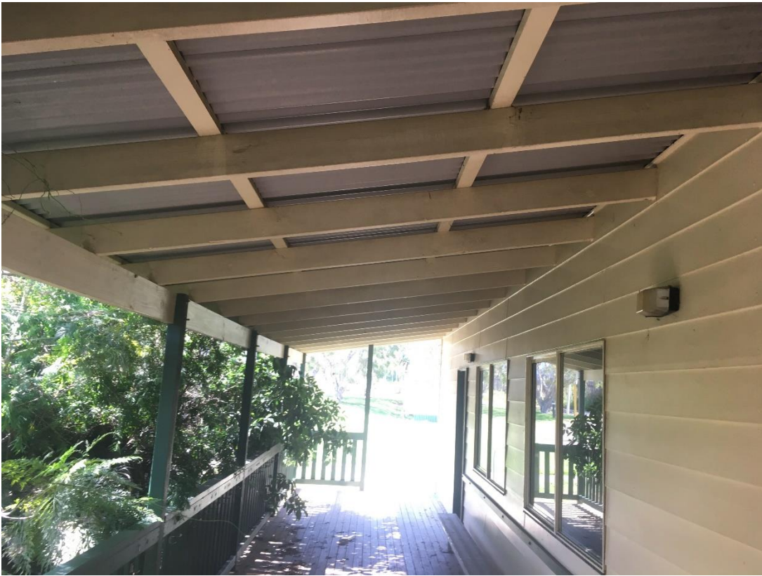
Plate 11: Wooden supports lining the roof. No evidence of bat activity was observed within this area
