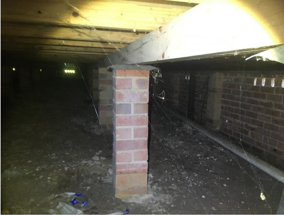
Plate 9: Space beneath one of the two buildings to be demolished. Large amount of spider webs suggesting nothing is flying through this area.
