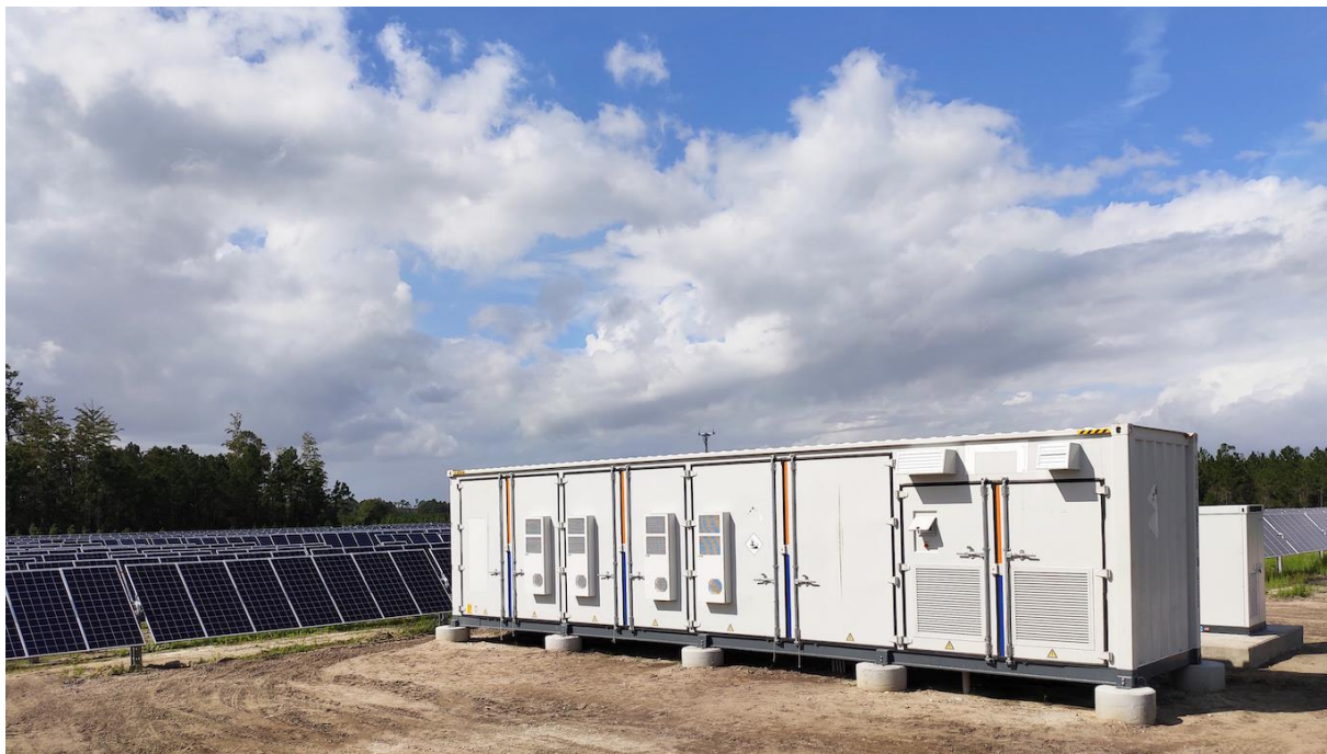
Image 4: Close up of example of battery unit with inverter adjacent to solar panels – for illustrative purposes only
