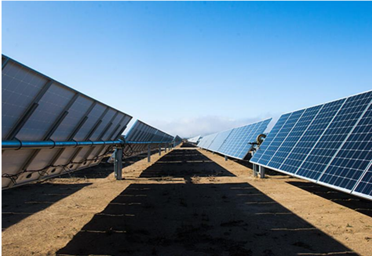
FIGURE 2 EXAMPLE OF TRACKING SOLAR PV PANELS
