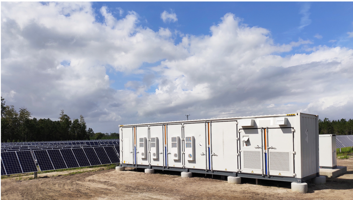
Image 2: Close up of example of battery unit with inverter adjacent to solar panels
