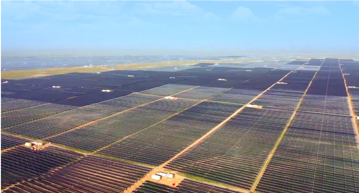
Image 1: Illustrative of battery units distributed throughout a solar farm
