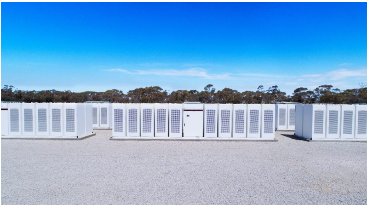
Image 2: Close up of example of battery units
