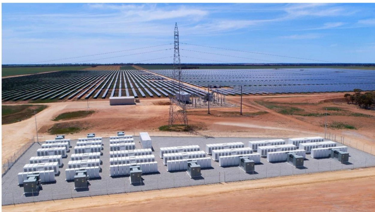
Figure 2-1: Image of a BESS coupled with a solar farm, with white battery units (for illustration purposes only)
