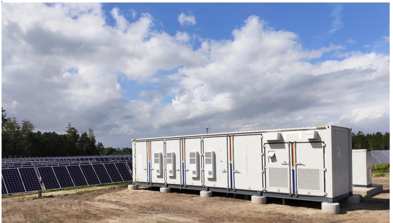
Figure 2-4: Close up image of battery unit with inverter adjacent to solar panels, with white battery units (for illustration purposes only)
