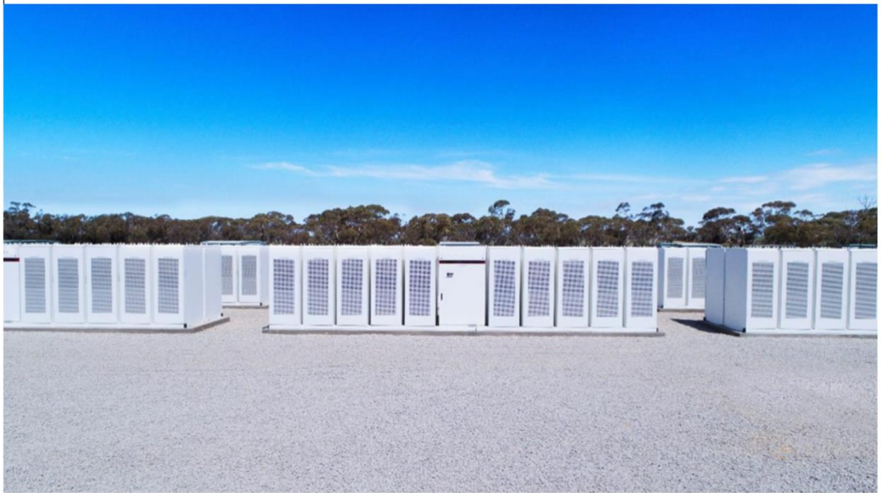
Figure 2-2: Close image of a centralised BESS, with white battery units (for illustration purposes only)
