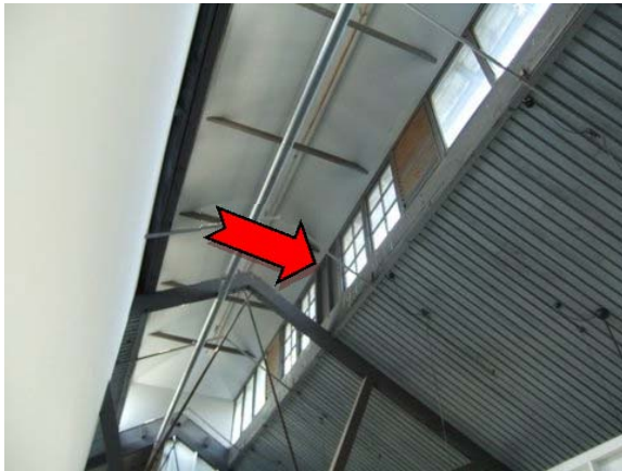
Photo 1. Level 4, interior, the loft, window infill panels – asbestos-containing fibre cement sheeting.
