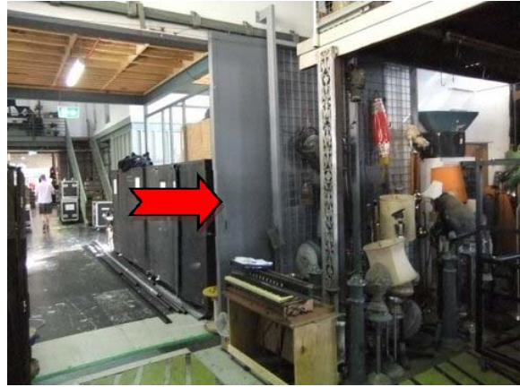
Photo 8. Level 3, interior, prop room – SMF-containing fire door core.
