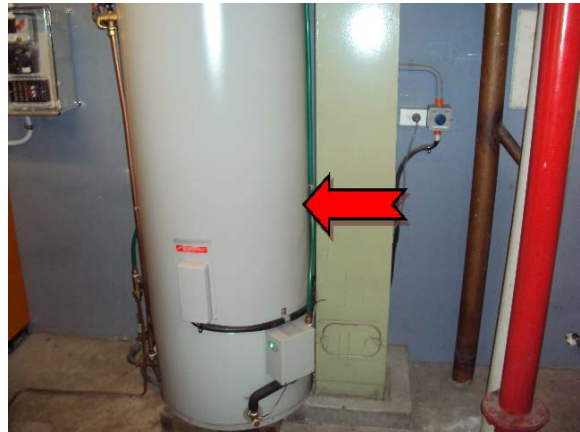
Photo 10. All levels, throughout, hot water heaters - suspected internal SMF insulation
