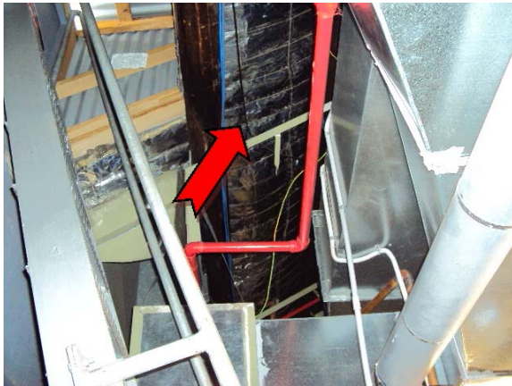
Photo 9. All levels, throughout, ceiling - suspected SMF sarking insulation
