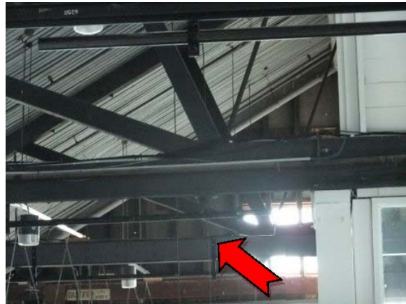
Photo 2. Level 3, interior, restaurant, gable infill panels - suspected asbestos-containing fibre cement sheeting.
