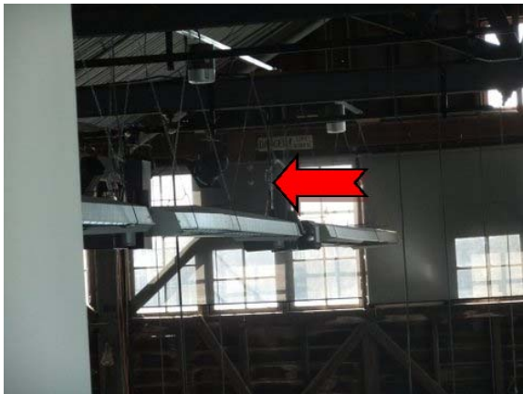
Photo 3. Level 3, interior, restaurant - asbestos-containing infill panels under windows.
