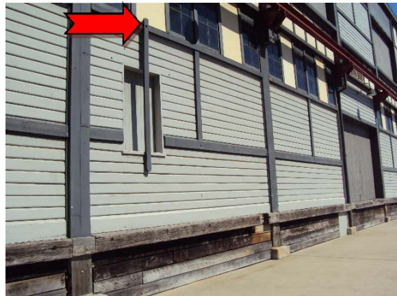
Photo 4. All levels, throughout, external and internal - asbestos containing infill panels around windows
