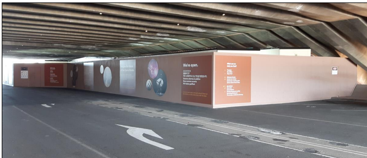
Figure 13 - Proposed Vehicle Concourse Main Site Compound with Lunch Rooms, Change Rooms, Ablutions, First Aid and Decking Area (JST set up shown)
