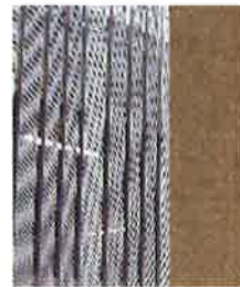
6 - LOUVRES - CAR PARK
