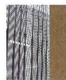
6 - LOUVRES - CAR PARK
