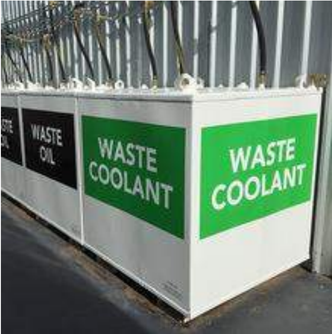
Figure 10: ARS Tank Storage System
