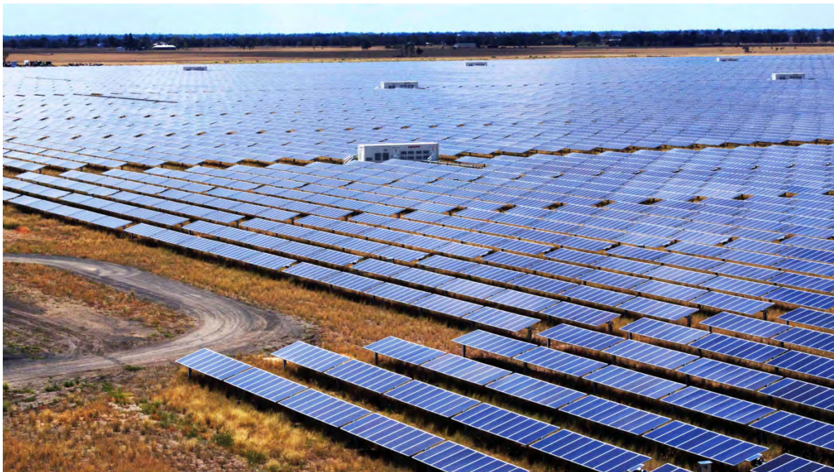
Photograph 2.2 Example of typical PV solar arrays for the approved project comprising single PV solar panels along tracking rows
