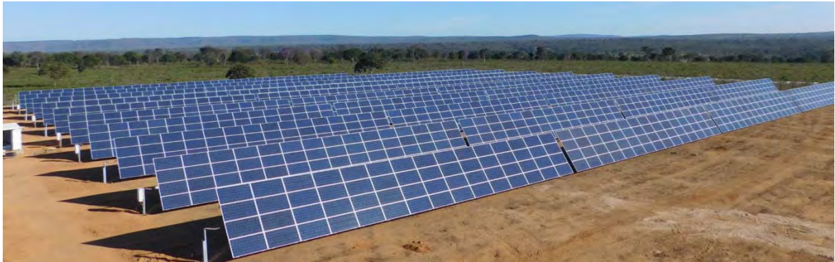
Photograph 2.3 Example of typical arrangement of PV solar panel arrays for the proposed modification – typical tracker rows comprising four PV solar panels orientated in a landscape arrangement along the length of the row
