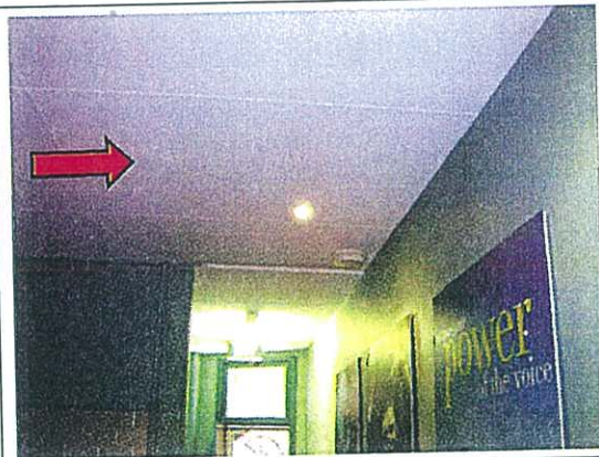
Photo 4. Ceiling, Reception room, Level 1, Sydney Choir Rehearsal – Asbestos fibre-cement sheeting
