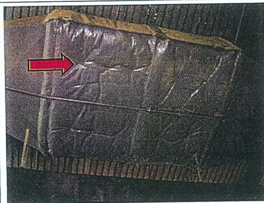
Photo 7. SMF insulation to air conditioning ductwork throughout building.
