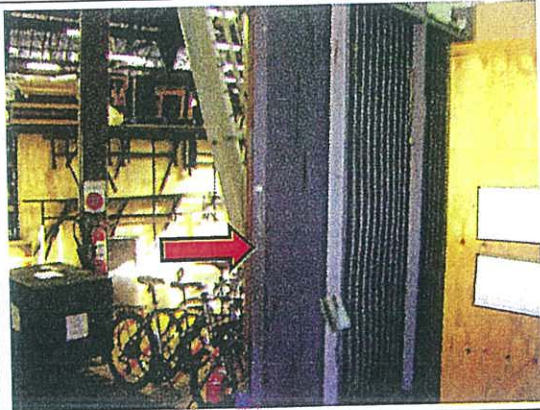
Photo 2. Sliding fire door, Workshop entrance, Level 3 – Suspected Asbestos fire door core
