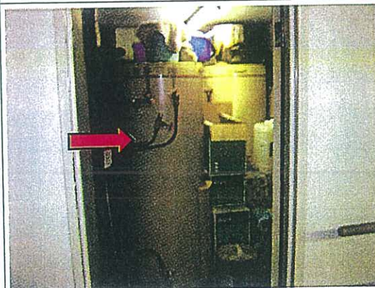
Photo 9. Suspected SMF material within Hot water heaters throughout building.
