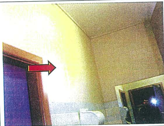
Photo 3. Walls, Male and Female Toilets, Level 1, Sydney Choir Rehearsal – Asbestos fibre-cement sheeting
