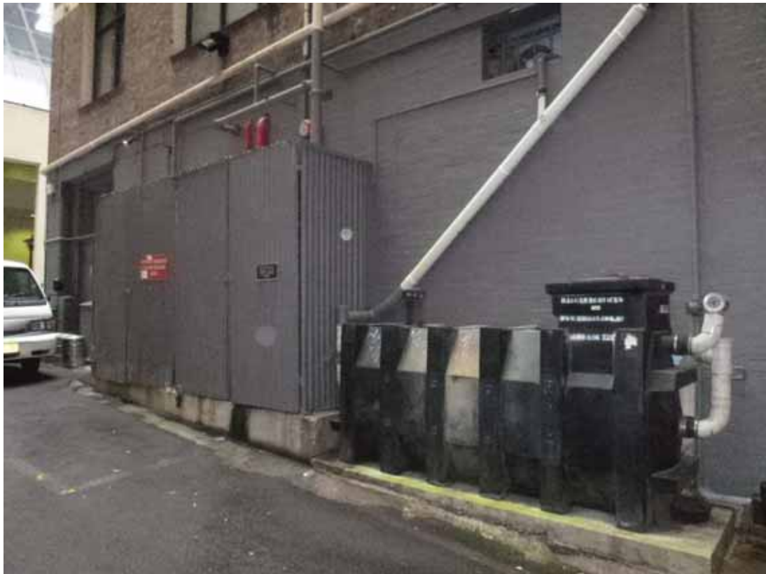
Plate 31: Grease trap (black structure) and sprinkler system (within metal enclosure, left of grease trap) at ground level, outside of Registered Club building
