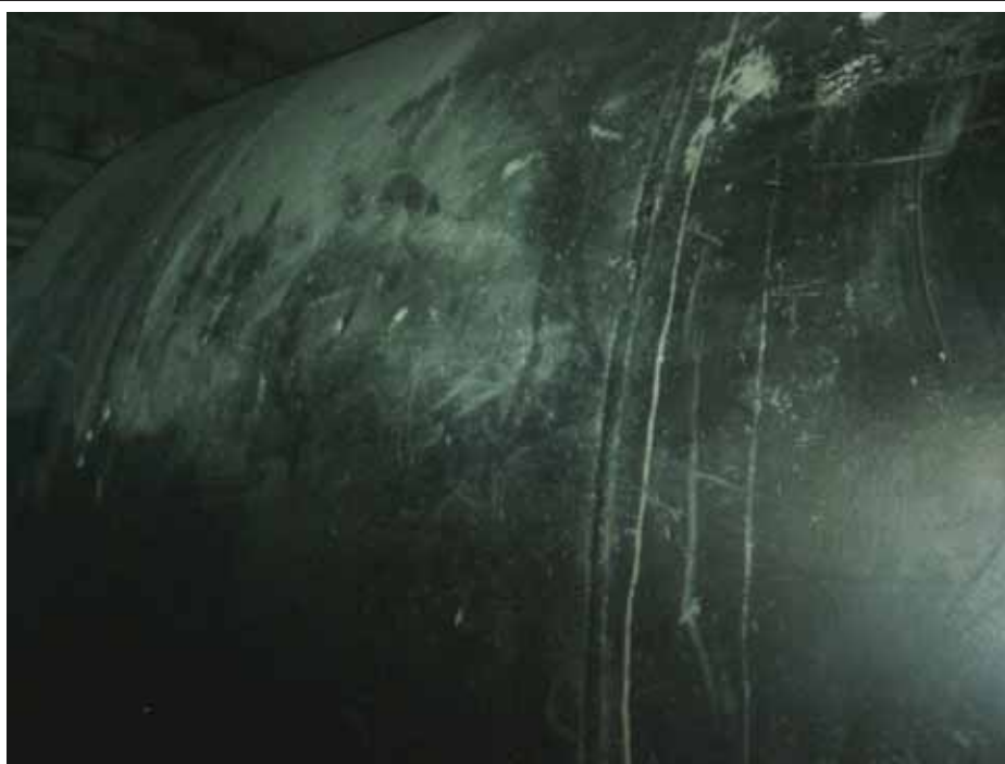
Plate 12: Closer veiw of decommisioned above ground tank within small concrete room in Lower Basement Level of Goldfields House Building
