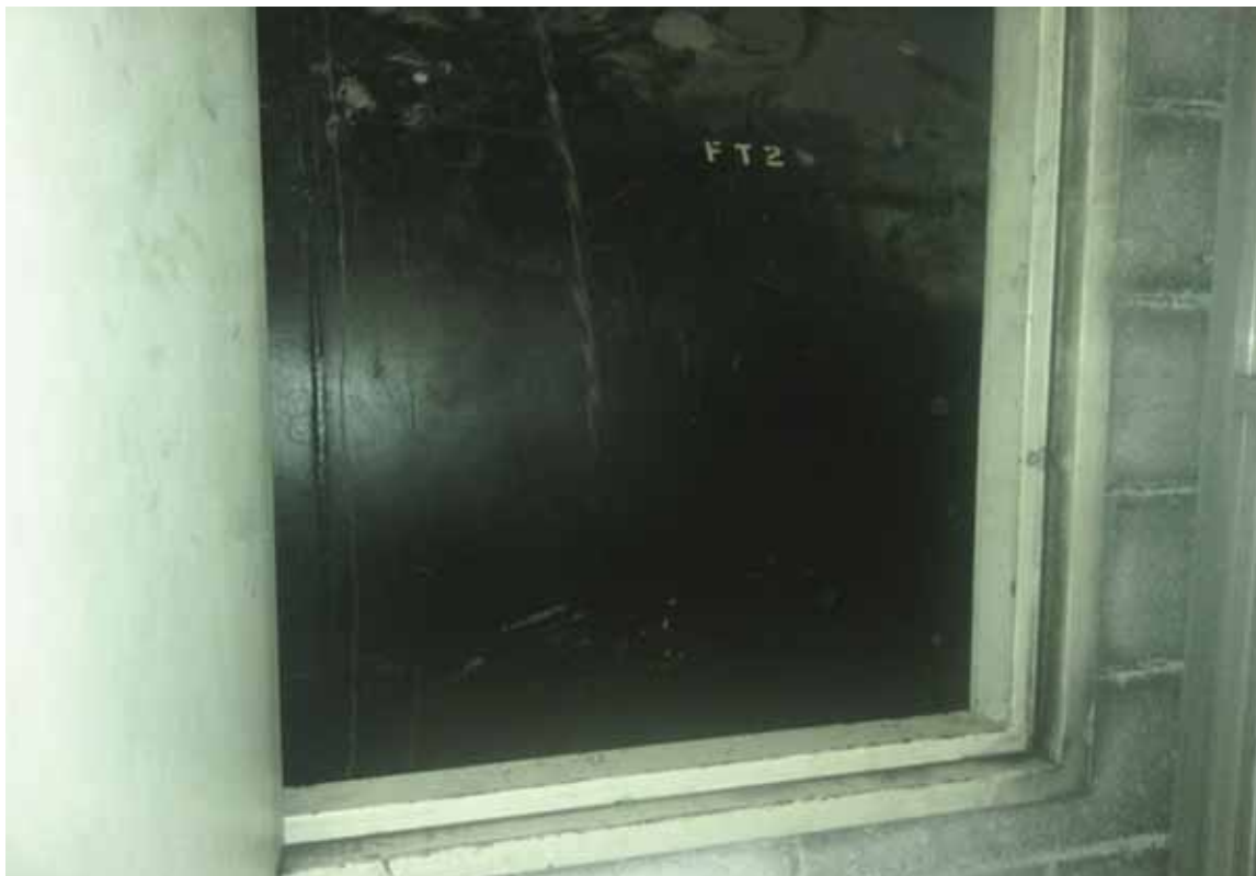
Plate 11: Decommisioned above ground tank within small concrete room in Lower Basement Level of Goldfields House Building
