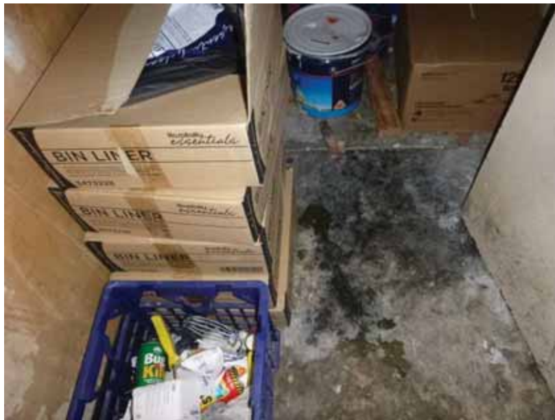
Plate 30: Staining on floor of cleaners storage room at ground level of Registered Club building
