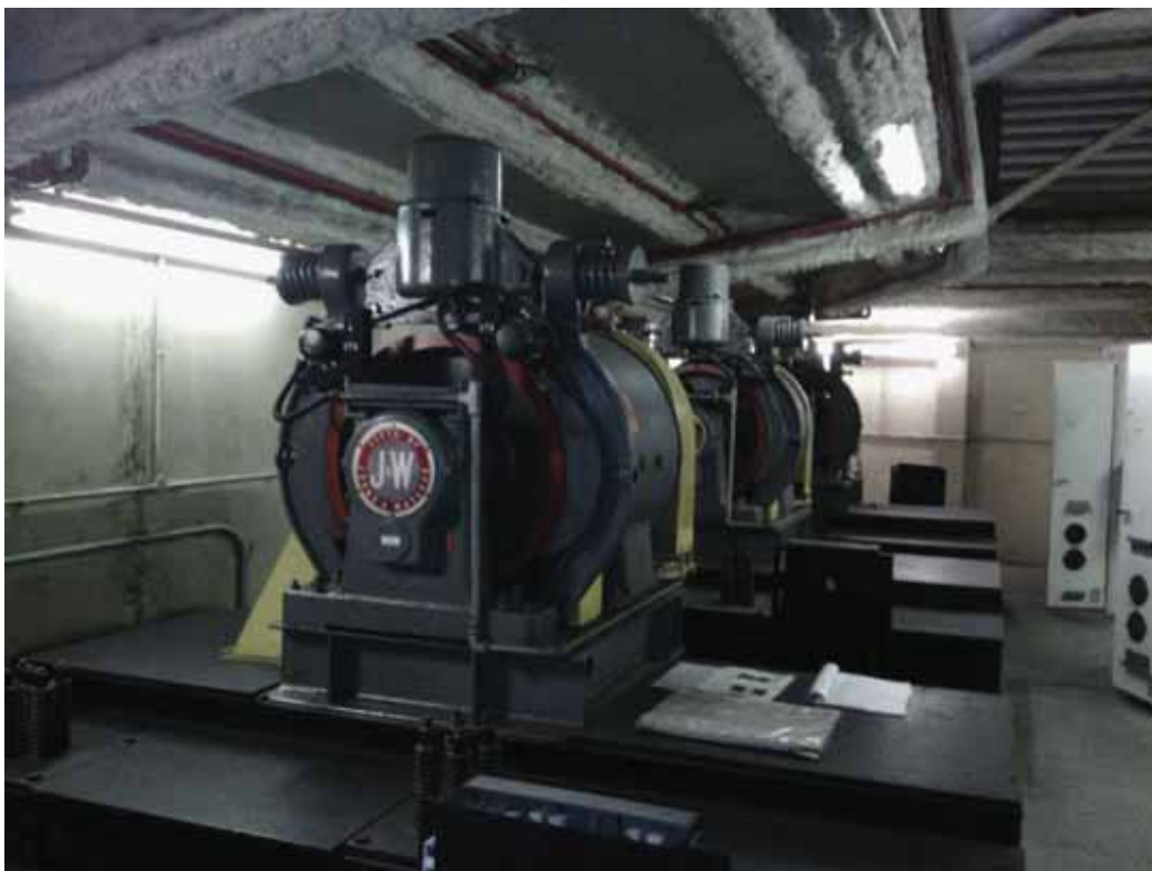
Plate 26: Lift Motor Room (LMR) at level 16 of Fairfax House Building
