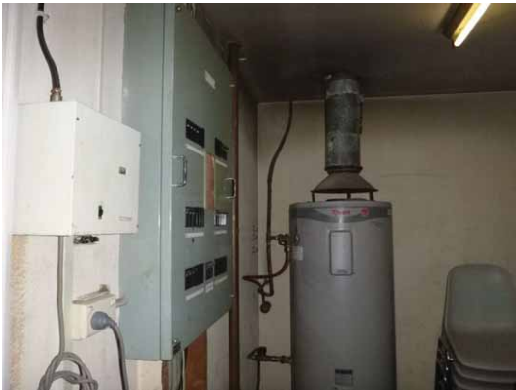
Plate 32: Boiler and electrical switchboard at level 6 of Registered Club building
