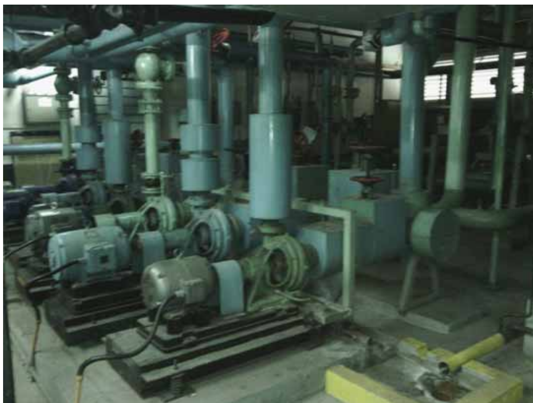
Plate 24: Plant Room of level 15 of Fairfax House Building
