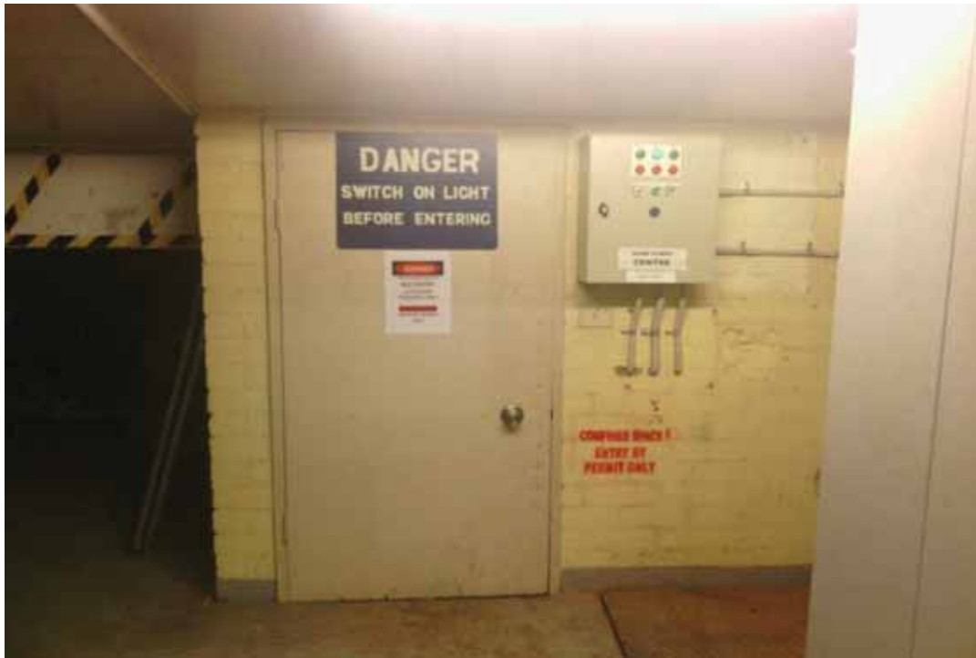
Plate 15: Substation in Lower Basement Level of Goldfields House Building
