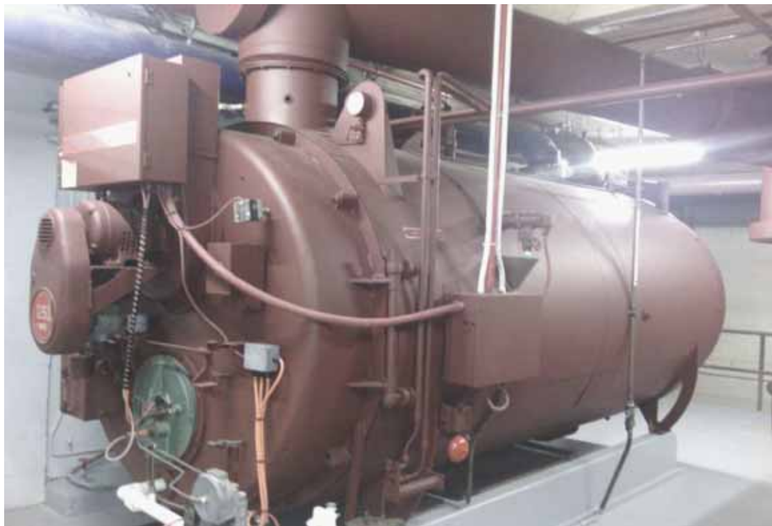
Plate 18: Boilers at Level 27 of Goldfields House Building
