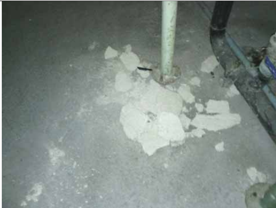
Plate 25: Flaked off ceiling material on the floor of the Plant Room of level 15 of Fairfax House Building
