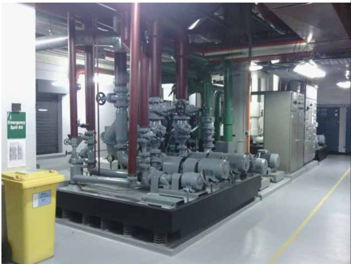
Plate 16: Chillers within Level 26 of Goldfields House Building
