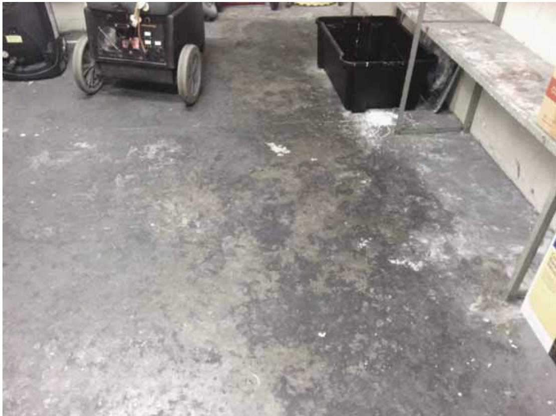
Plate 9: Staining observed in the cleaners room at the Basement Level at the Goldfields House
