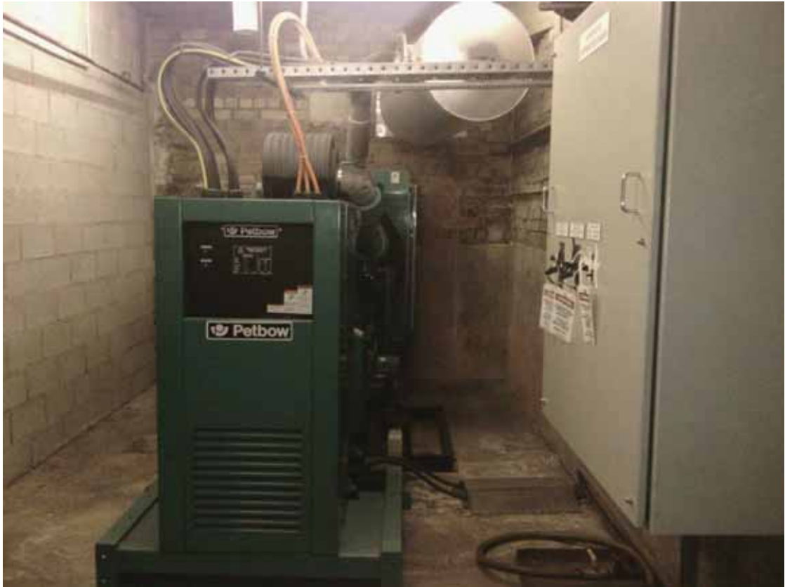
Plate 13: Decommisioned deisel generator in Lower Basement Level of Goldfields House Building
