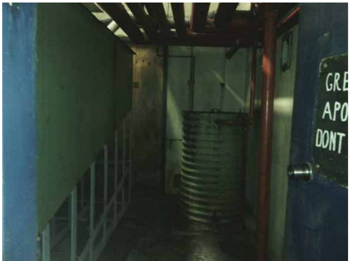
Plate 10: Grease Trap Room at Basement Level of the Goldfields House Building
