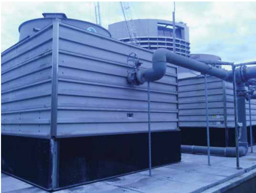
Plate 20: Cooling Towers at rooftop level 28 of Goldfields House
