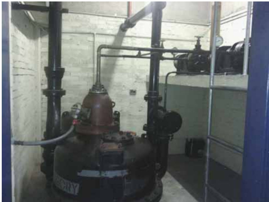
Plate 14: Sewerage Ejector in Lower Basement Level of Goldfields House Building
