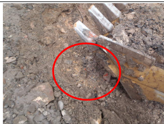
Photo 13. Stockpile 225, Excavation Area – Presumed asbestos-containing fibre cement fragments
