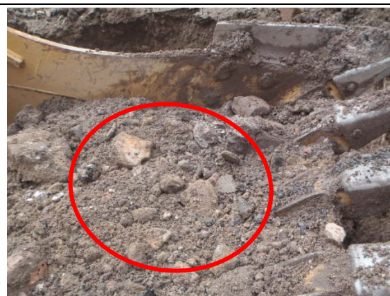
Photo 15. Stockpile 225, Excavation Area – Presumed asbestos-containing fibre cement fragments
