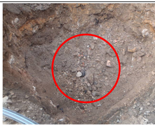
Photo 16. Stockpile 225, Excavation Area – Presumed asbestos-containing fibre cement fragments
