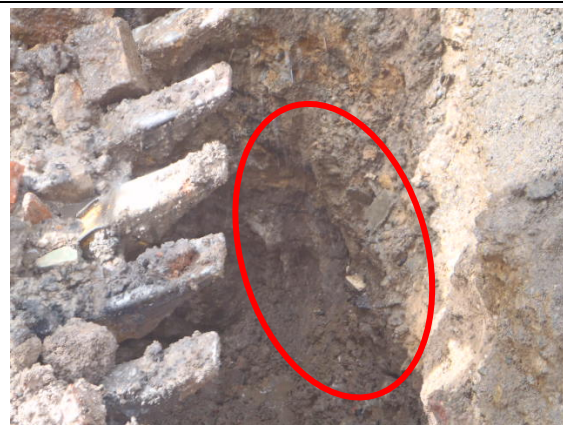
Photo 17. Stockpile 225, Excavation Area – Presumed asbestos-containing fibre cement fragments
