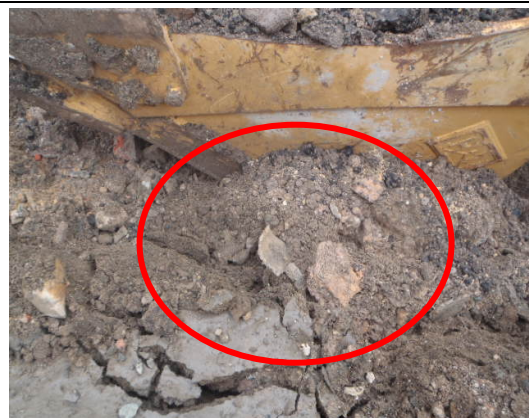
Photo 12. Stockpile 225, Excavation Area – Presumed asbestos-containing fibre cement fragments
