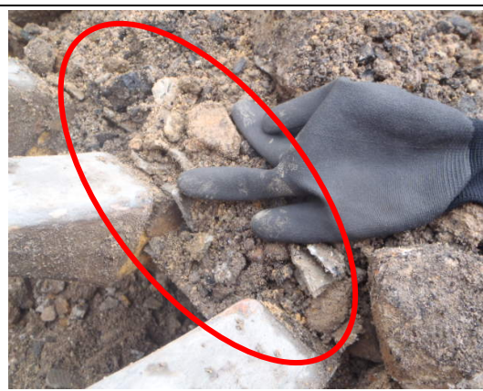
Photo 14. Stockpile 225, Excavation Area – Presumed asbestos-containing fibre cement fragments
