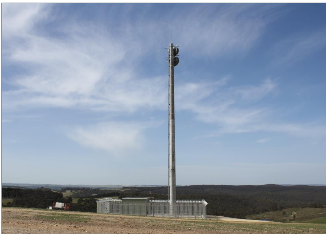
Figure 5-5 An example of a microwave communications tower from Gullen Range Wind Farm
