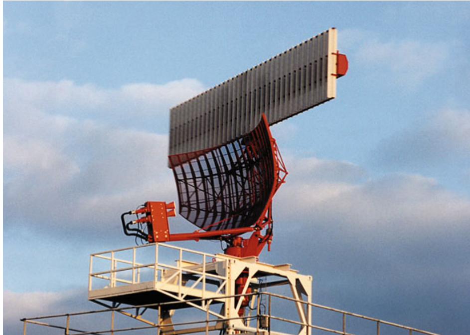
Figure 4: Primary and secondary co-mounted radar antennas
