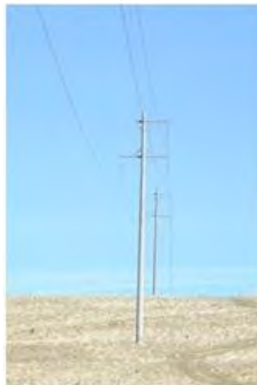
132kV single circuit concrete poles
