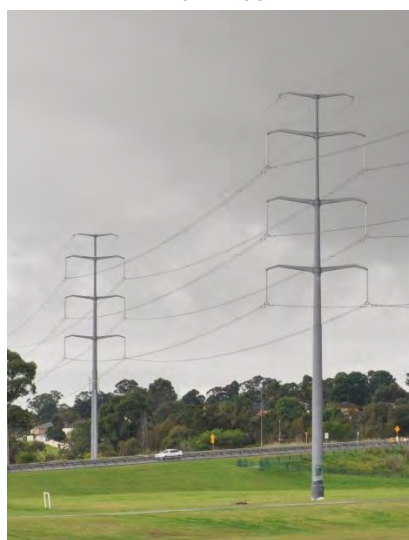
330kV double circuit steel poles
