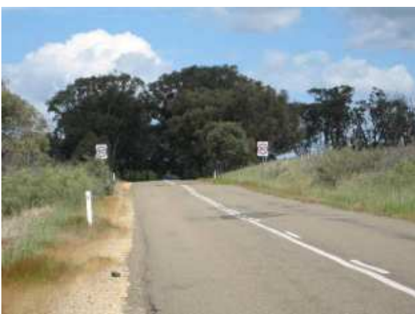
PLATE 17 Burrinjuck Road failing pavement
