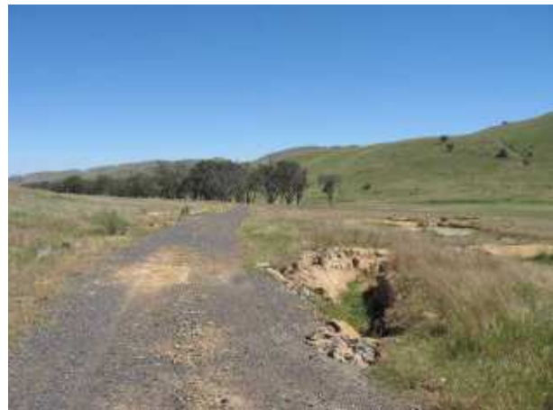
PLATE 52 Whitefields Road erosion at 3.33km.
