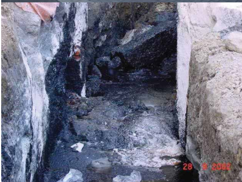
Figure 3.20: Tar contamination apparently uncovered during construction works in September 2002. Mark Burns, Lend Lease (Millers Point)
