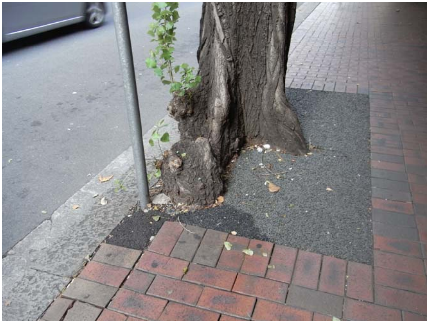
Photograph 2: Tree # 6 - Illustrating the evidence of conflict between tree's roots and adjacent kerb and footpath paving.
