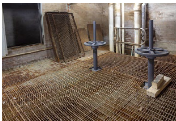
Figure 4.6: Access to the Water-Cooling Manifold (Curio 2020)
