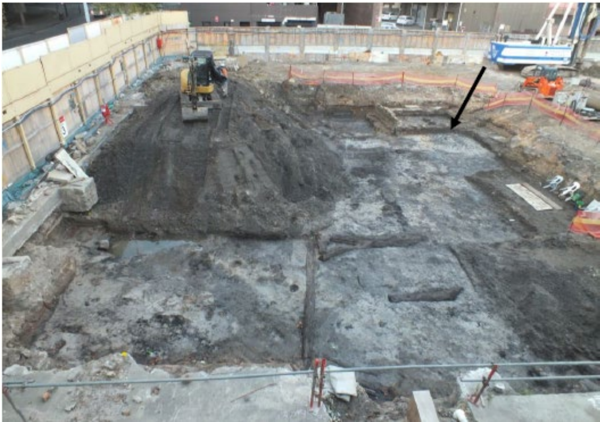
Figure 7.11: Earliest phase on site with an 1840s cottage in good condition (Source: AMC 2015)
