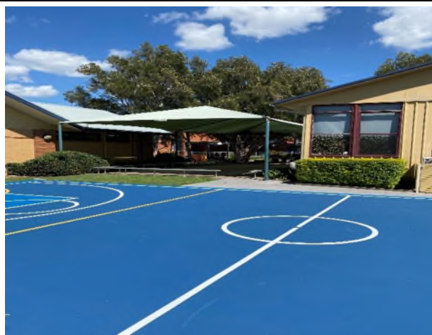
Photograph 2: View west from the eastern perimeter boundary. Basketball court surface conditions
