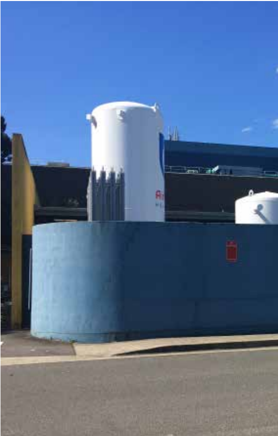
Fig 27: View of bulk oxygen supply
