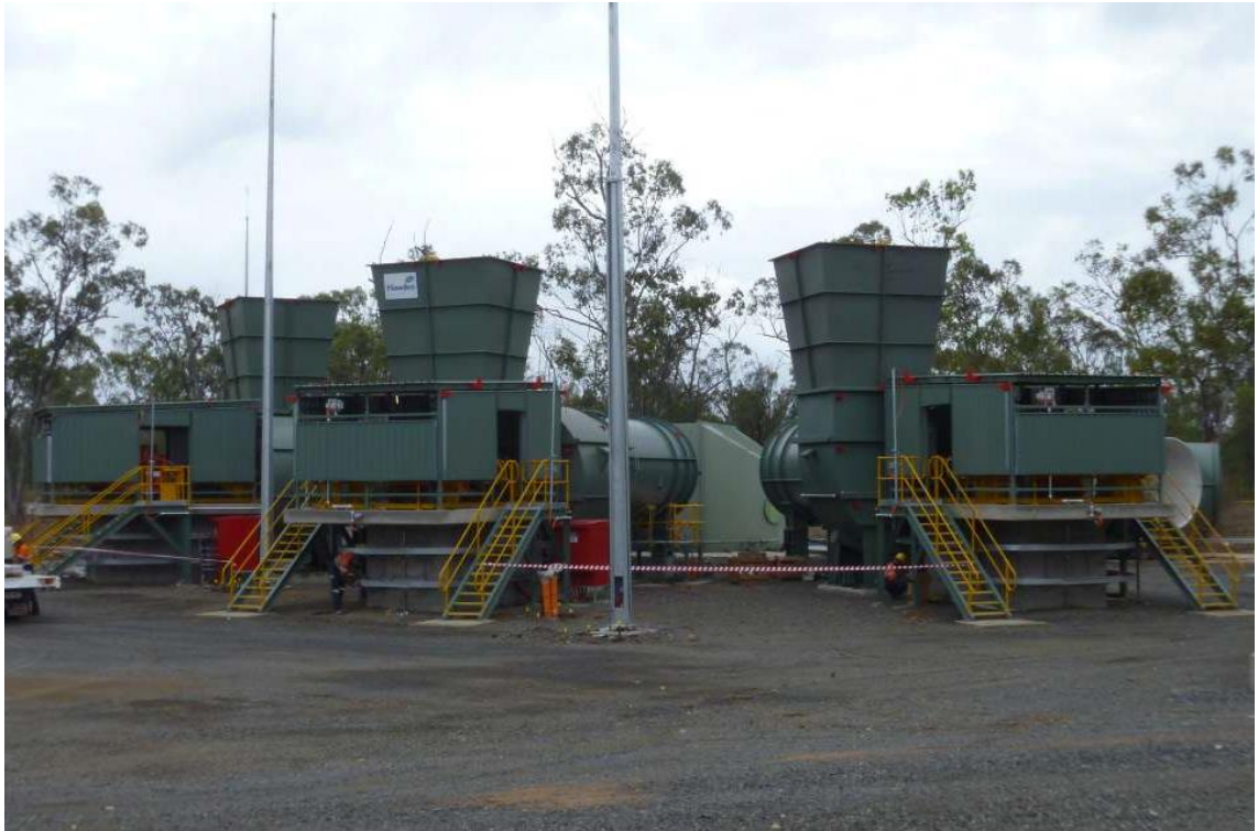
Photograph 3-1 Example of triple vertical ventilation fans and housing
