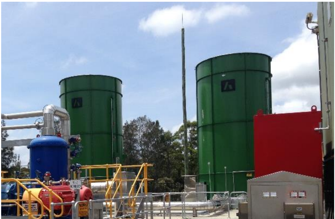
Photograph 3-2 Example of gas flares
