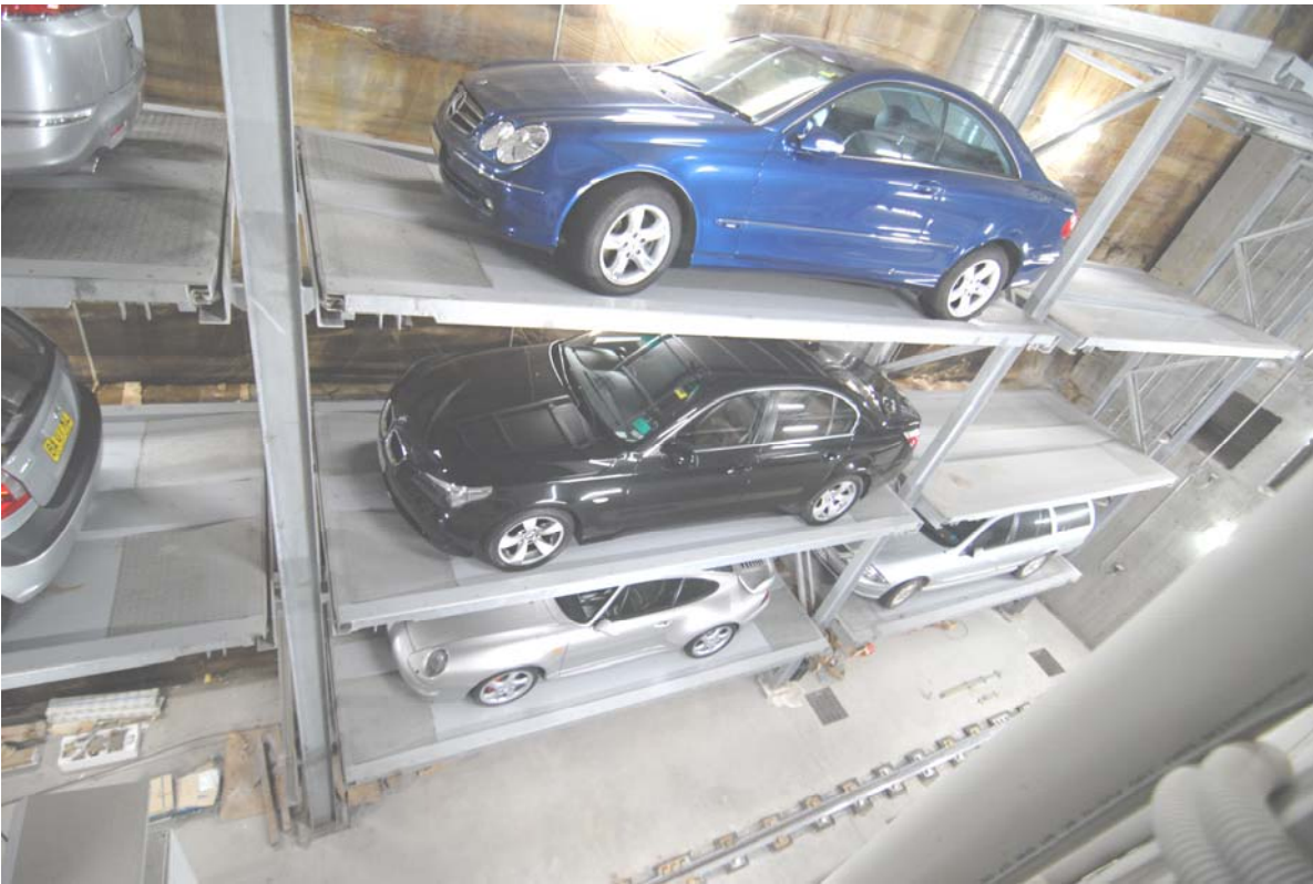
Figure 10.01 – automatic car parking system
