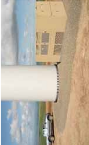
Generator Transformer (Source: Infigen Energy)
