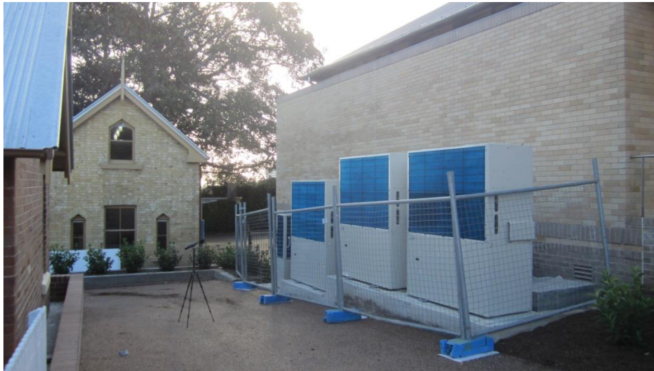
Figure 4: New Mechanical plant (Condensers units next to the multi activity centre) during the noise measurements
