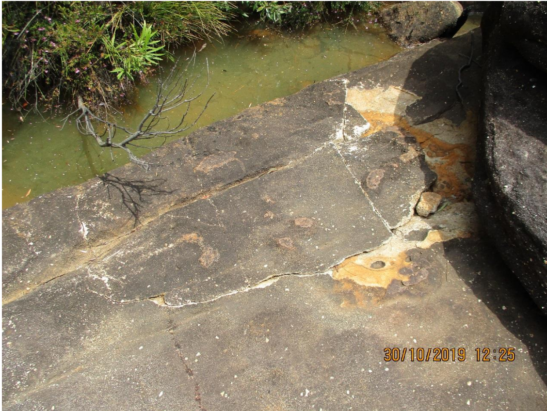
Plate 18: Eastern Tributary, MRIP08, Photo Point 4, cracking – spring 2019.
