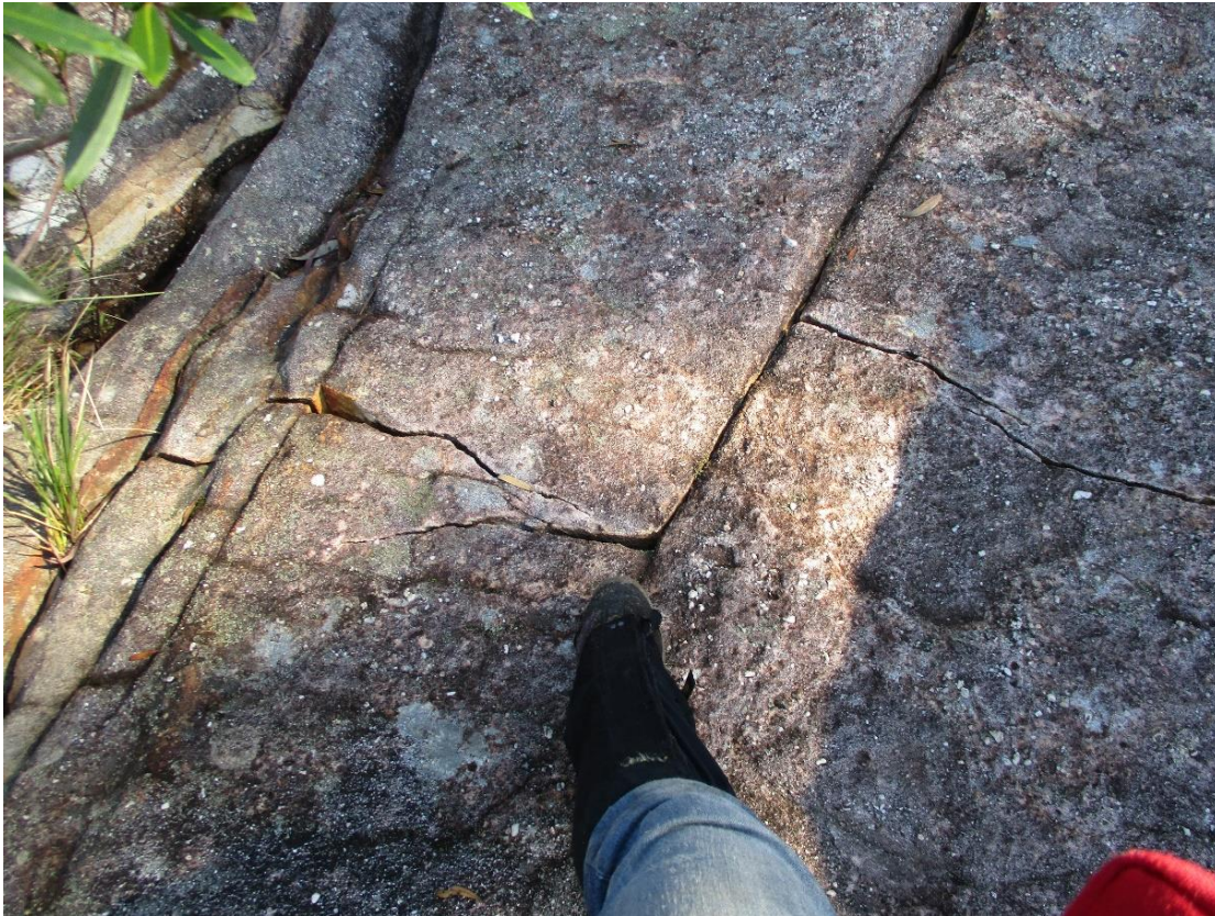
Plate 12: Eastern Tributary, MRIP08, Photo Point 8, cracking – autumn 2020.
