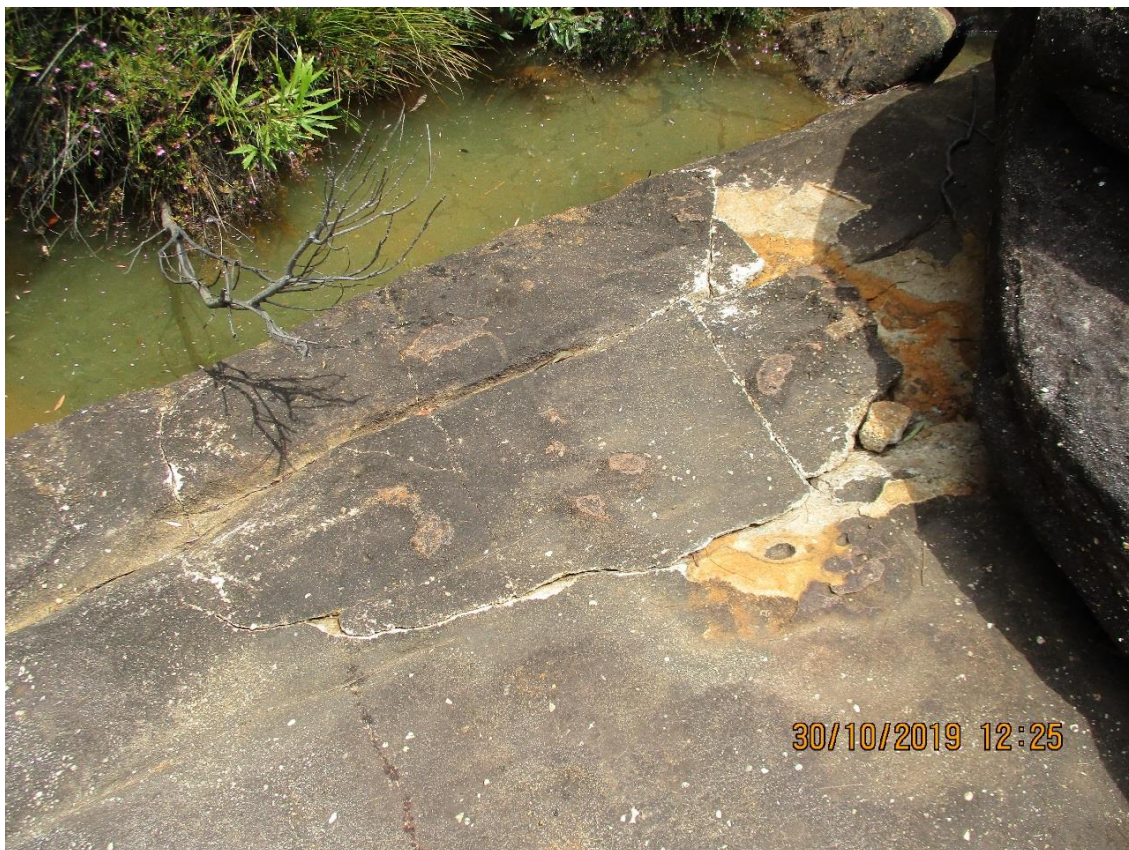
Plate 11: Eastern Tributary, MRIP08, Photo Point 4, cracking – spring 2019.
