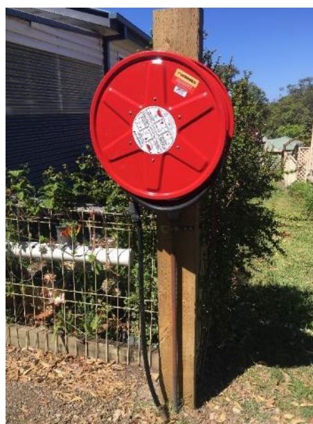
Plate 3.4 Hose reels located within existing caravan park
