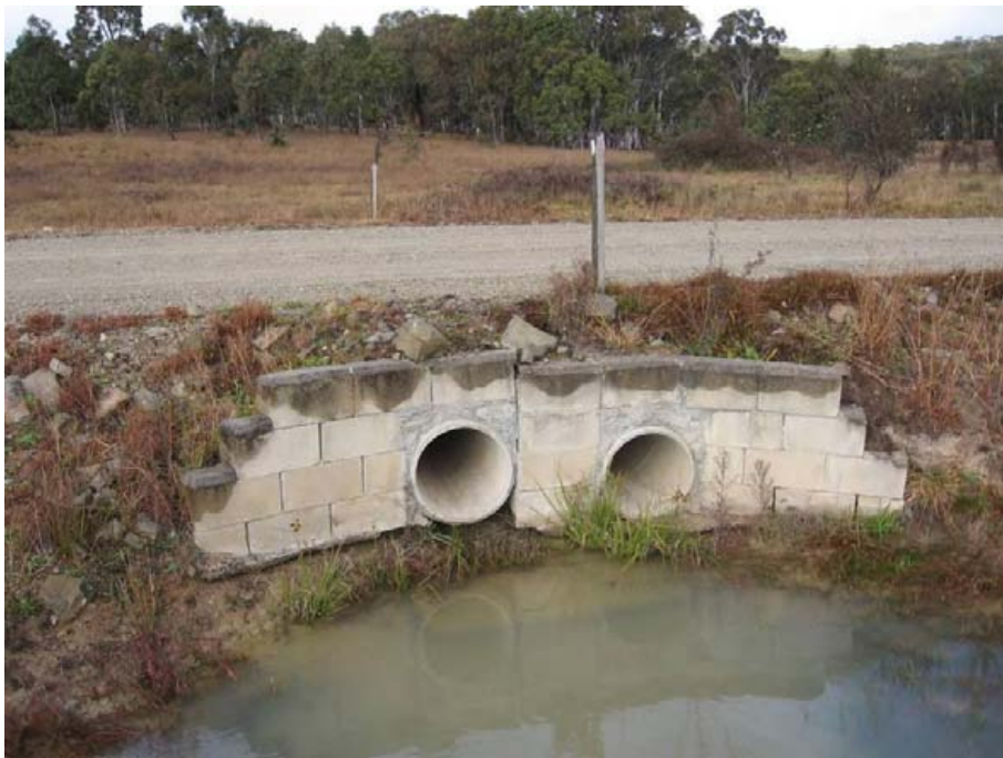
Figure 2-4 Canyonleigh Road faulty pipe culverts
