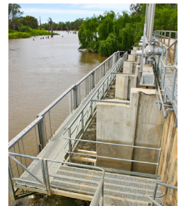
Bundidgerry Storage and Regulator
