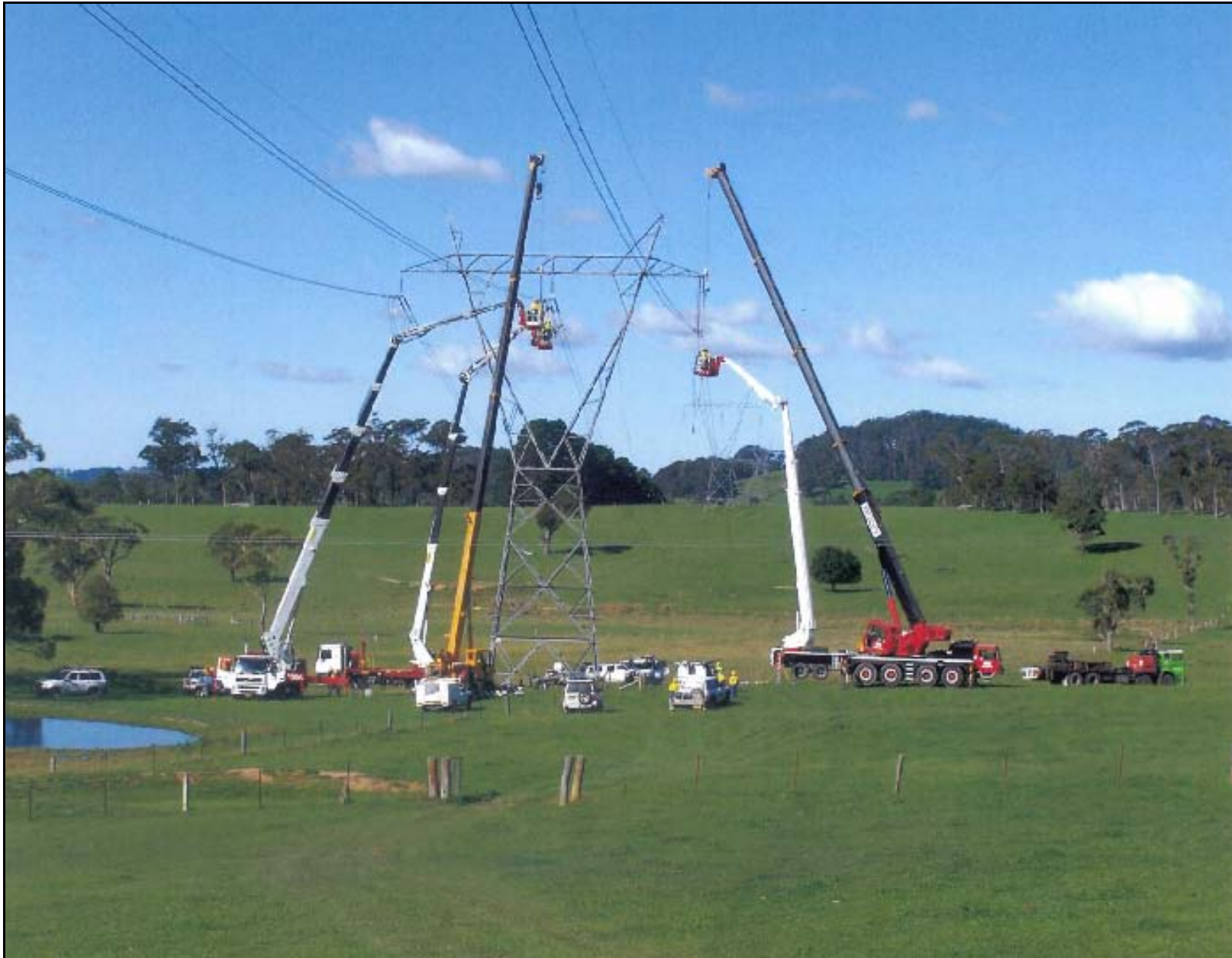
330kV Tower and Line
