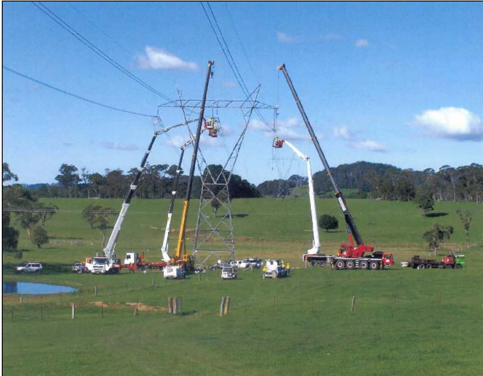
330kV Tower and Line
