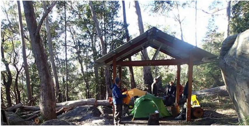
Structure established near 'the Ruined Castle' in Blue Mountains National Park for provision of rainwater for park visitors (shown here under construction)
