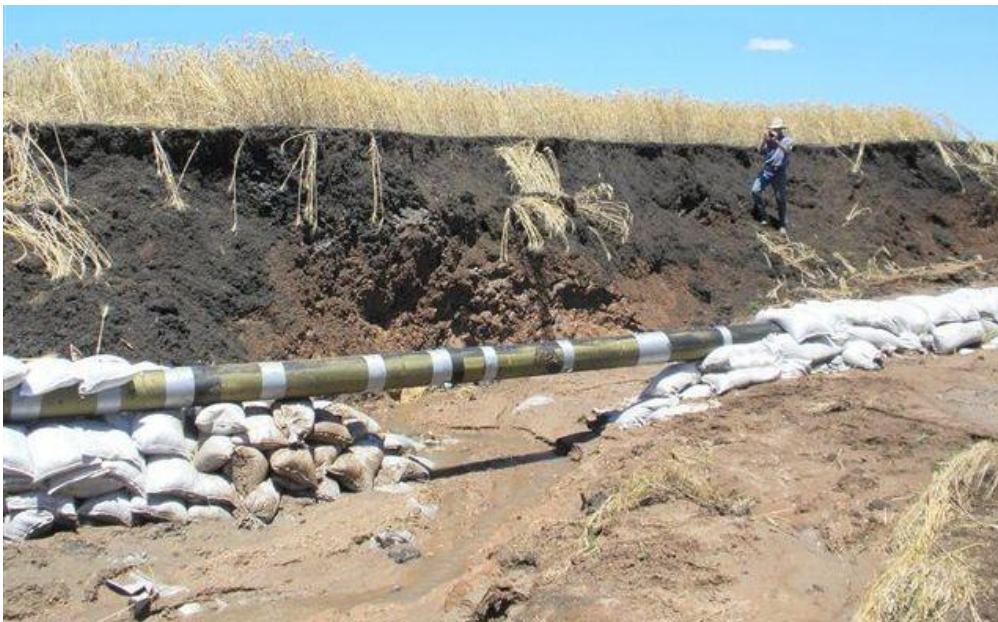
Photo 2: Gully and exposed pipe at Barana with failed sand bag supports
