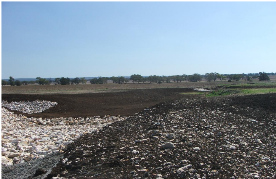
Photo 4: Looking downhill along rehabilitated pipe crossing failure at gully at “Barana”. Note natural gully width in right of mid ground.
