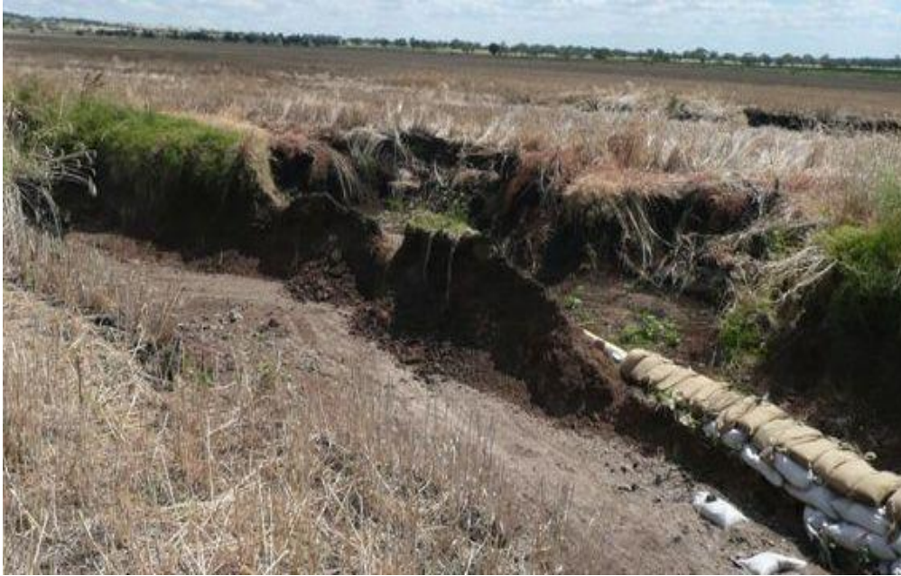
Photo 1: Gully and exposed pipe at Barana with spur gully following pipeline
