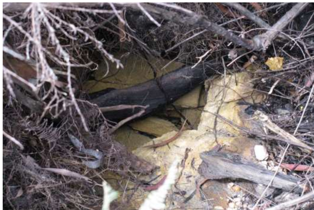
Photo 15: The same crack after the emergency minewater discharge from LDP004 had stopped.
