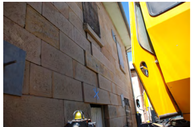
Figure 9: Indications of possible earlier out-of-plane movement of northern wall of Building 'B' suggested value of the mid-height monitoring of the wall.
