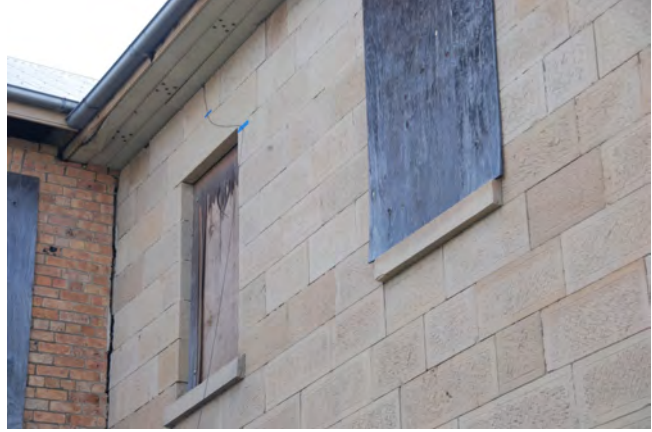
Figure 5: Single accelerometer placed at centre of rear wall of Building 'A' to gauge wall flexure. Note large crack separating stone wall from extension would have allowed independent movement.
