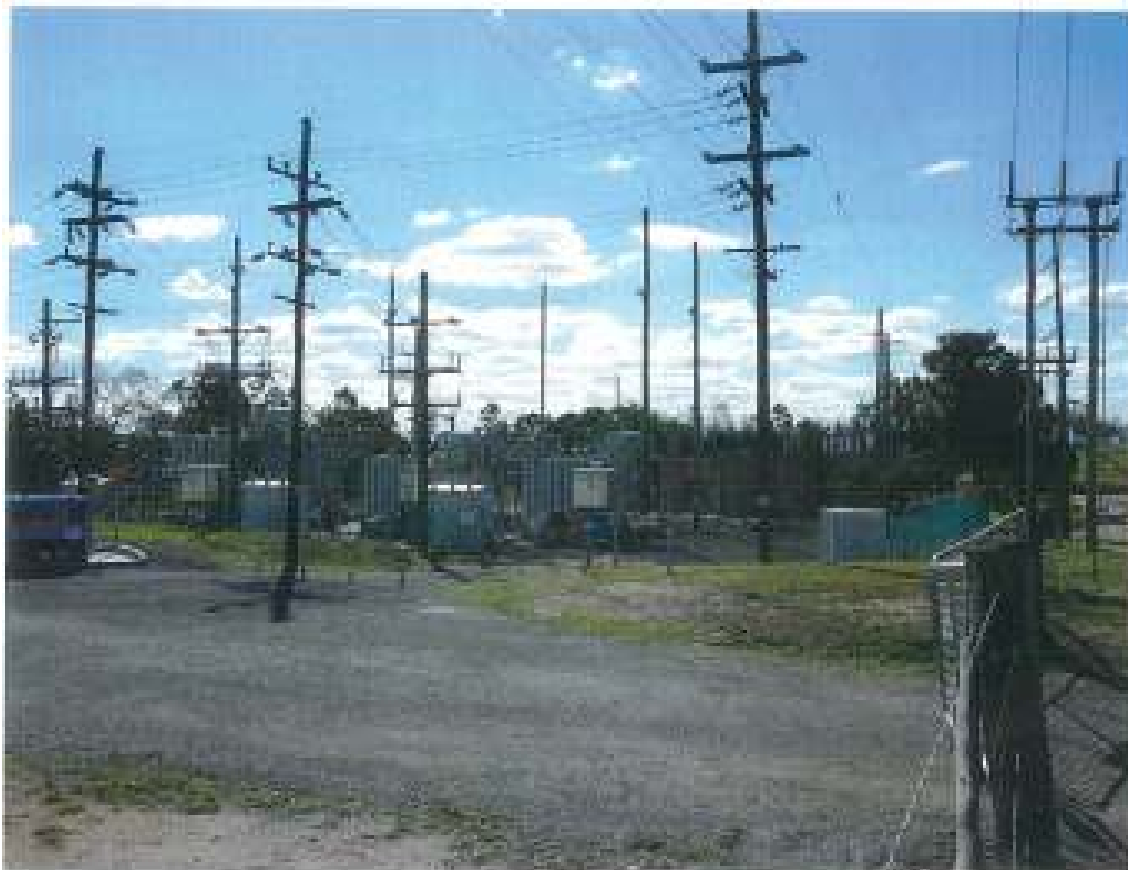
Plate 1: MTW Electrical Switchyard
