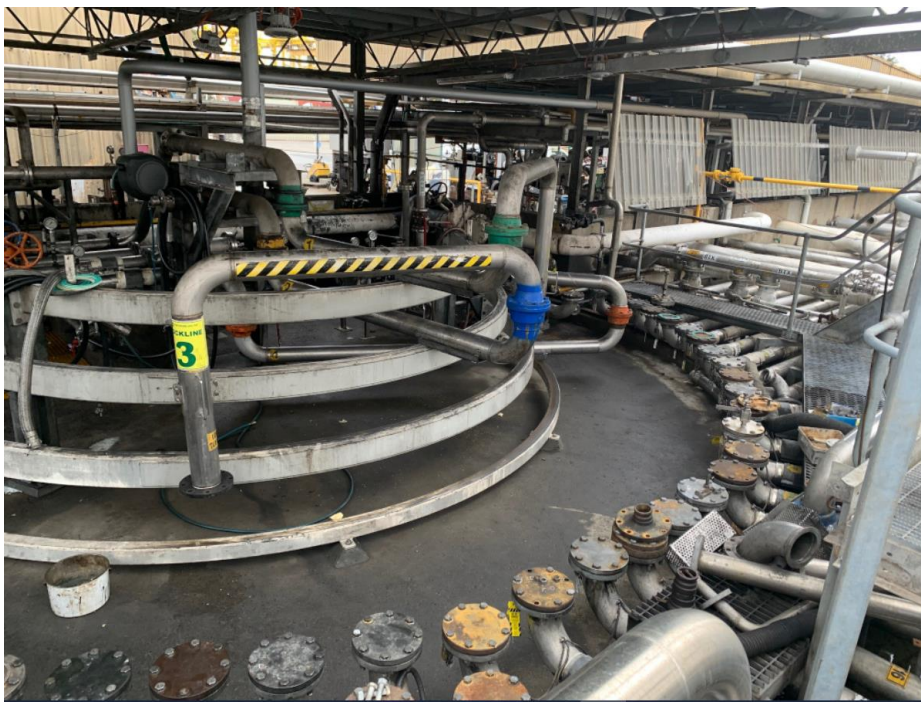
Main hose exchanger pit with roof over and weather protection shown for pumps top right
