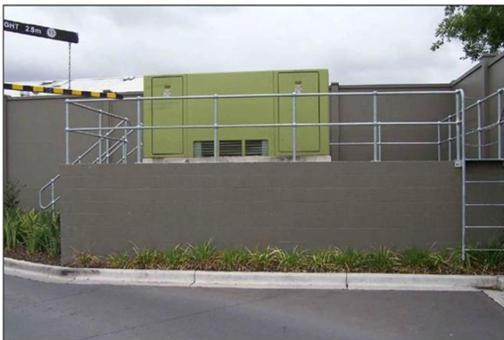
Figure 51 - Example substation raised above 1:100 flood level
